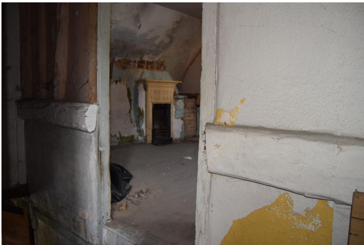
Plate 20: Cut tie-beam at head of staircase
