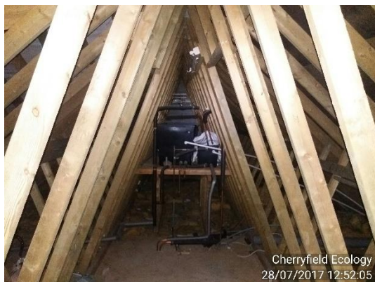
Figure 7: Bitumen felt to right and BRM to left
