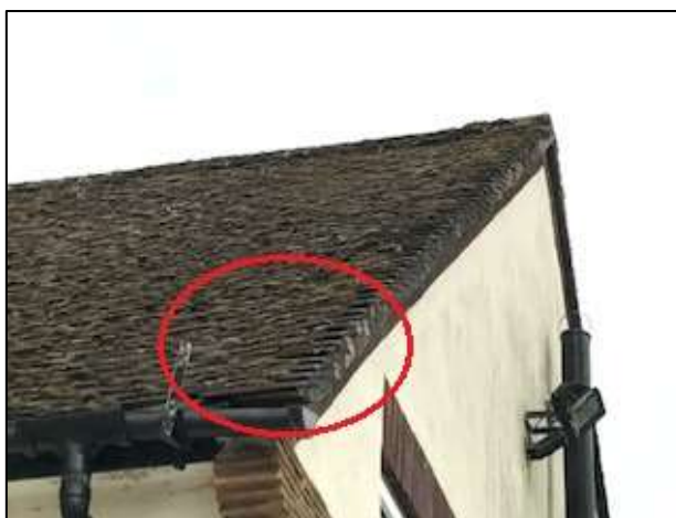
Photo 5: Examples of gaps in slates on south-west elevation roof.
