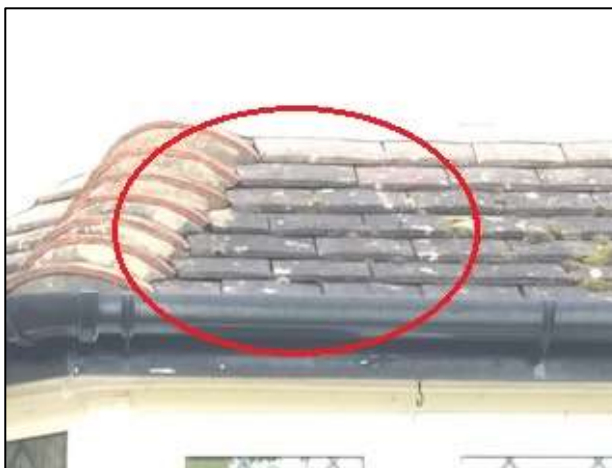
Photo 7: Close up photo of gaps in clay tiles above bay window.
