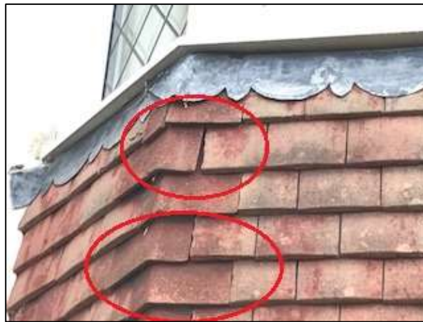
Photo 9: Close up photo of hanging tiles with gaps above first floor bay window on south-west elevation.
