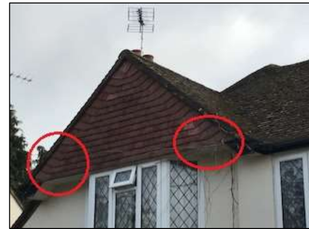
Photo 10: Hanging tiles above the first floor bay window on south-west elevation. Location of gaps in tiles circled.
