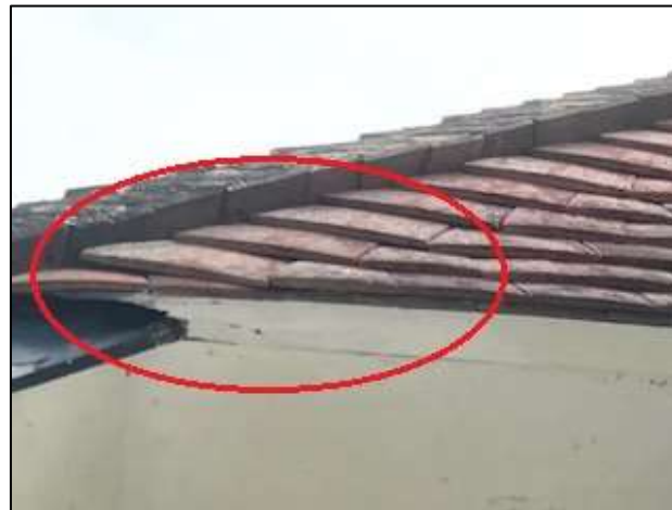
Photo 11: Close up photo of hanging tiles with gaps above first floor bay window on south-west elevation.
