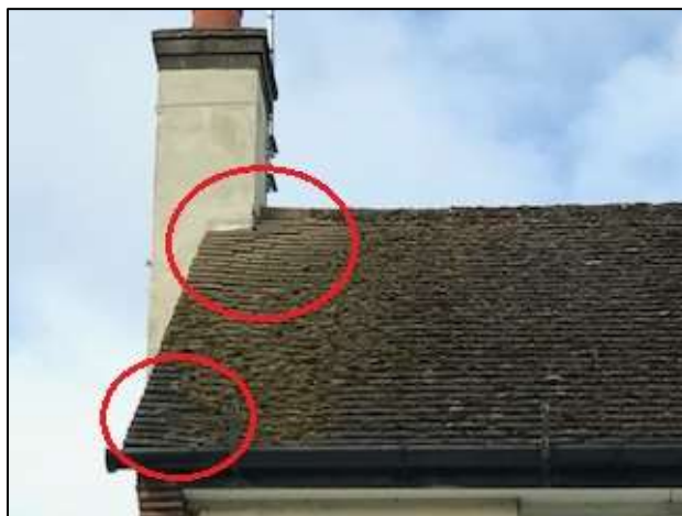
Photo 4: Sunken roof of southeast side of north-east elevation roof creating gaps in tiles below the chimney.
