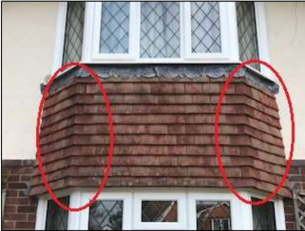
Photo 8: Hanging tiles above first-storey bay window on south-west corner elevation. Location of gaps in tiles circled.
