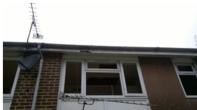
Plate 4.3: Broken Ceiling of Building 1.
