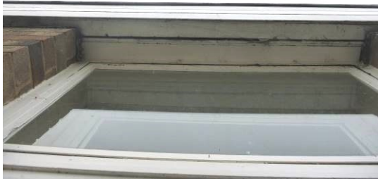
19. Gap between timbers above the kitchen window (Target note 1).
