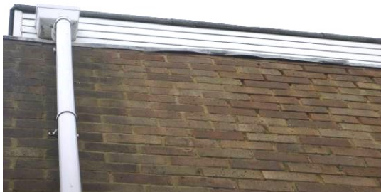
23. Warped metal on the southern side of building 4 (Target note 3).
