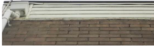
22. Warped metal on the western side of building 3 by the drain pipe (Target note 2).
