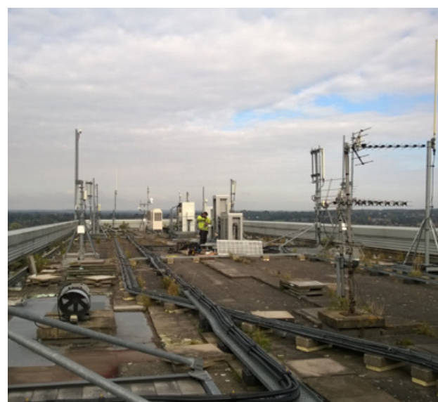
Existing communication masts and antenna
