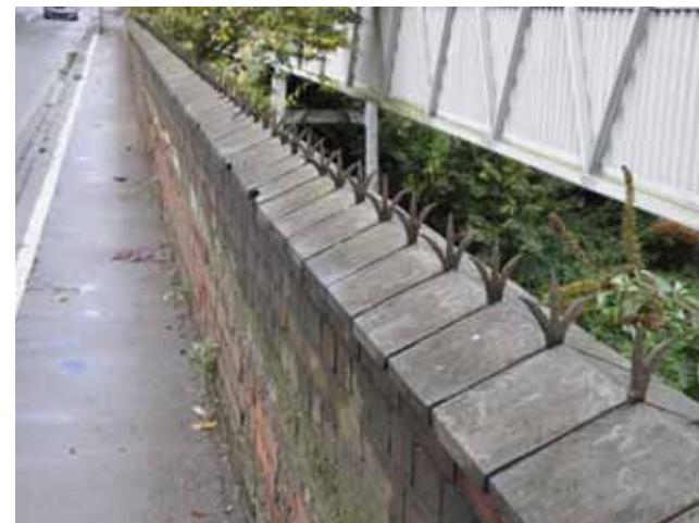
Figure 11: Detail of anti-climb spikes on low mileage parapet
