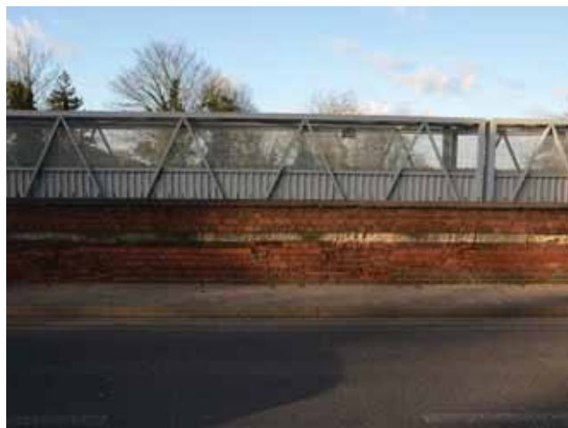
Figure 10: Detail of low mileage parapet
