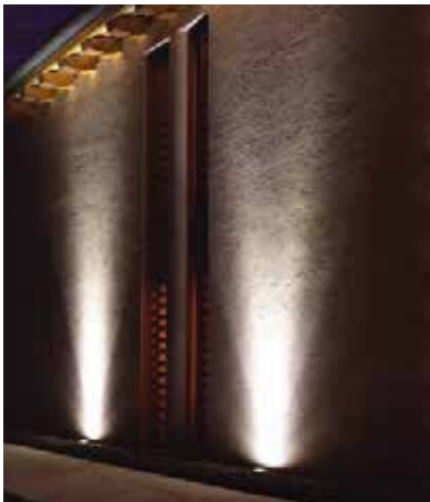
Feature Lighting Building Uplighter
