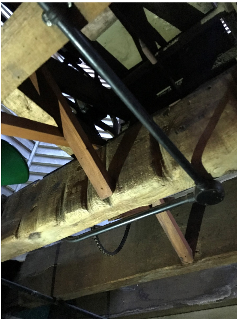
Plate 23: Wear on Joist at Original Hatch/Winch Location
