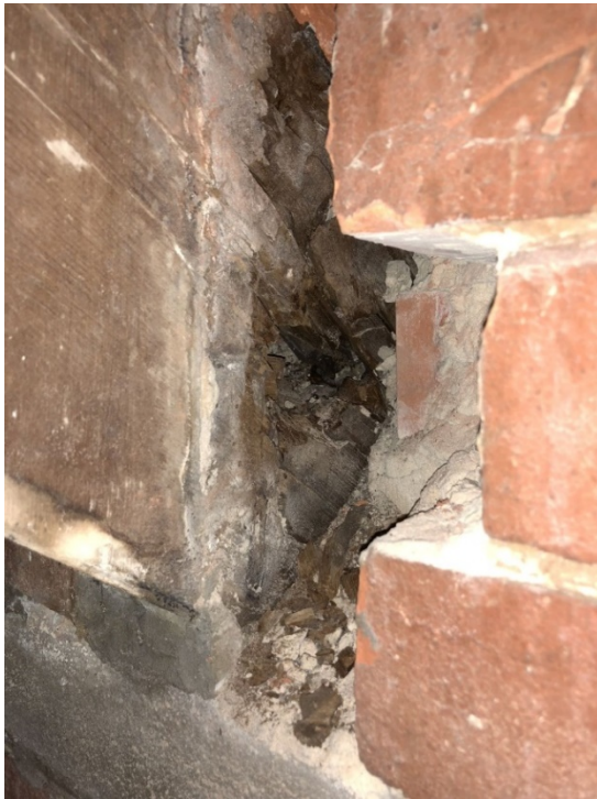
Plate 26: Example Damaged Truss End
