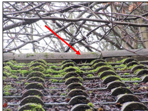
Photograph 22: Gap under ridge tile
