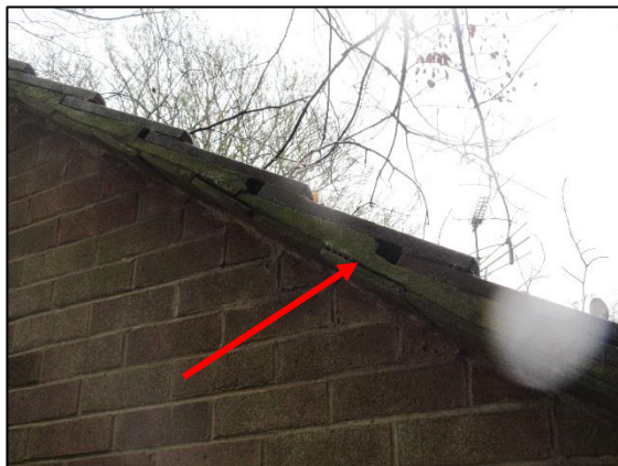
Photograph 23: Gaps under roof tiles
