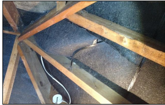
Photo 5: B1 damaged sarking
