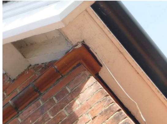
4. Gap at corner of front.
