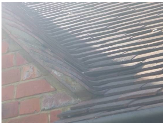
7. Gap at junction of rear pitched section
