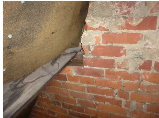
22. Gap at rear eaves space with wooden board exposed.
