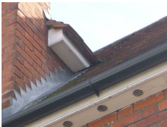
13. Gap under soffit at junction of chimney and roof.
