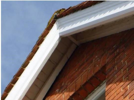
3. Gap under soffit of front gable.
