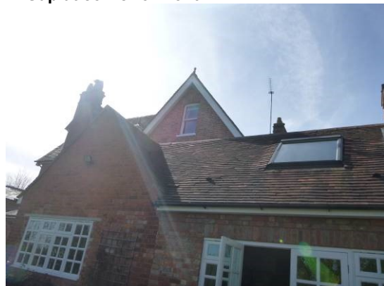
6. Occasional gaps beneath tiles in rear section.
