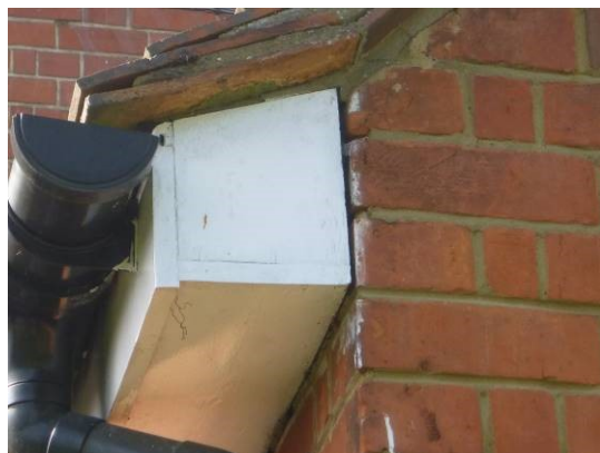
8. Gap beneath timber soffits.
