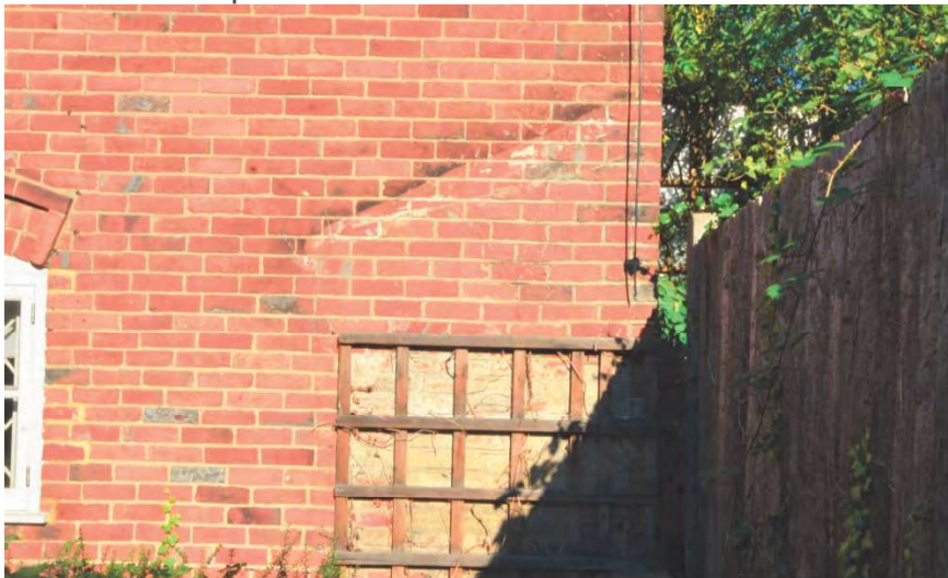
Plate 23: Scarring from former adjoining structure
