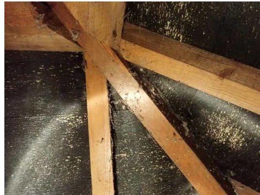
Photo 10 – Timberwork with cobwebs
