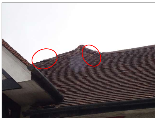
Photo 4 – Gaps to hip bonnets to front of house
