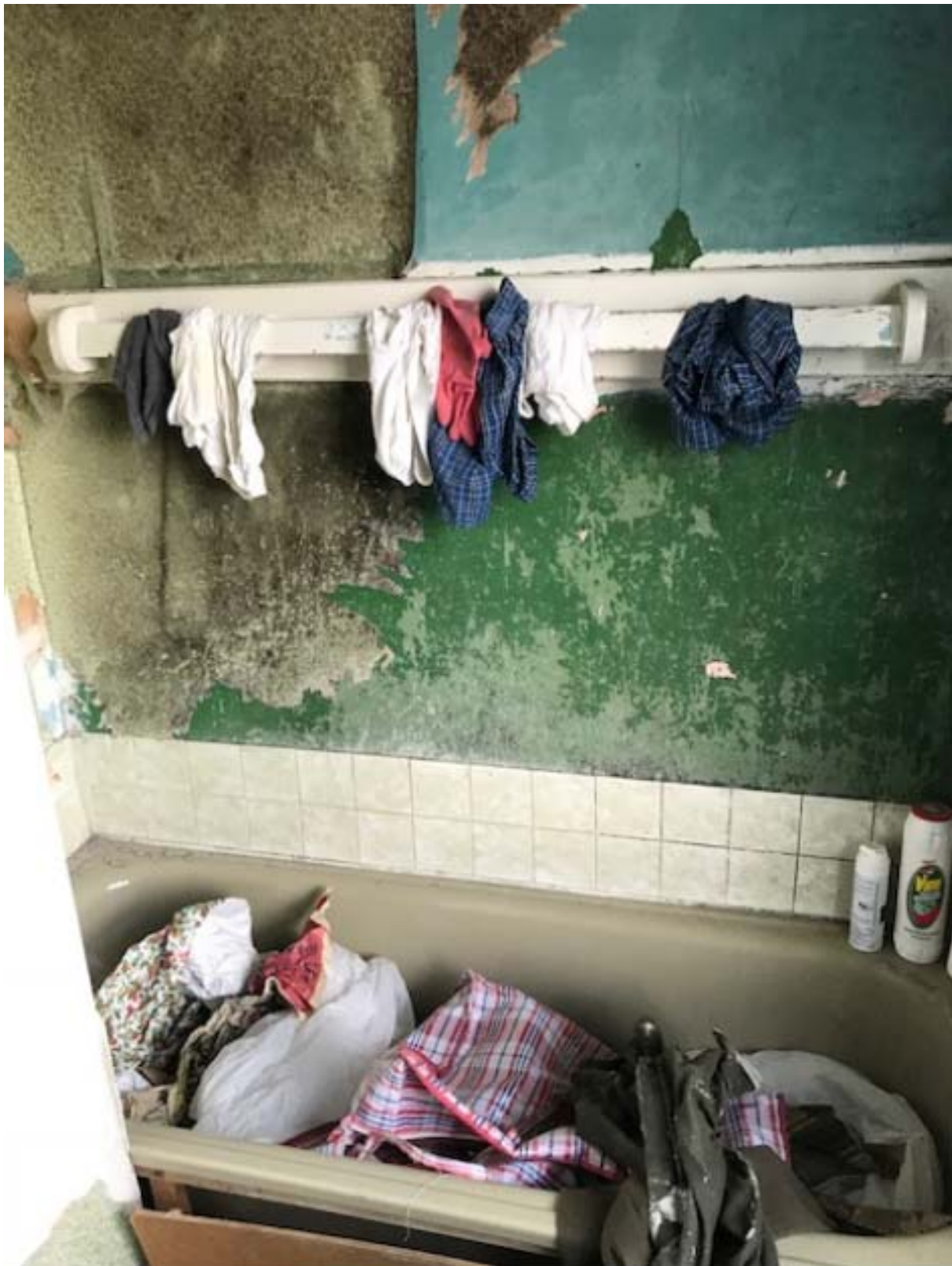
Fig A – Existing bathroom, damp on walls, peeling paintwork
