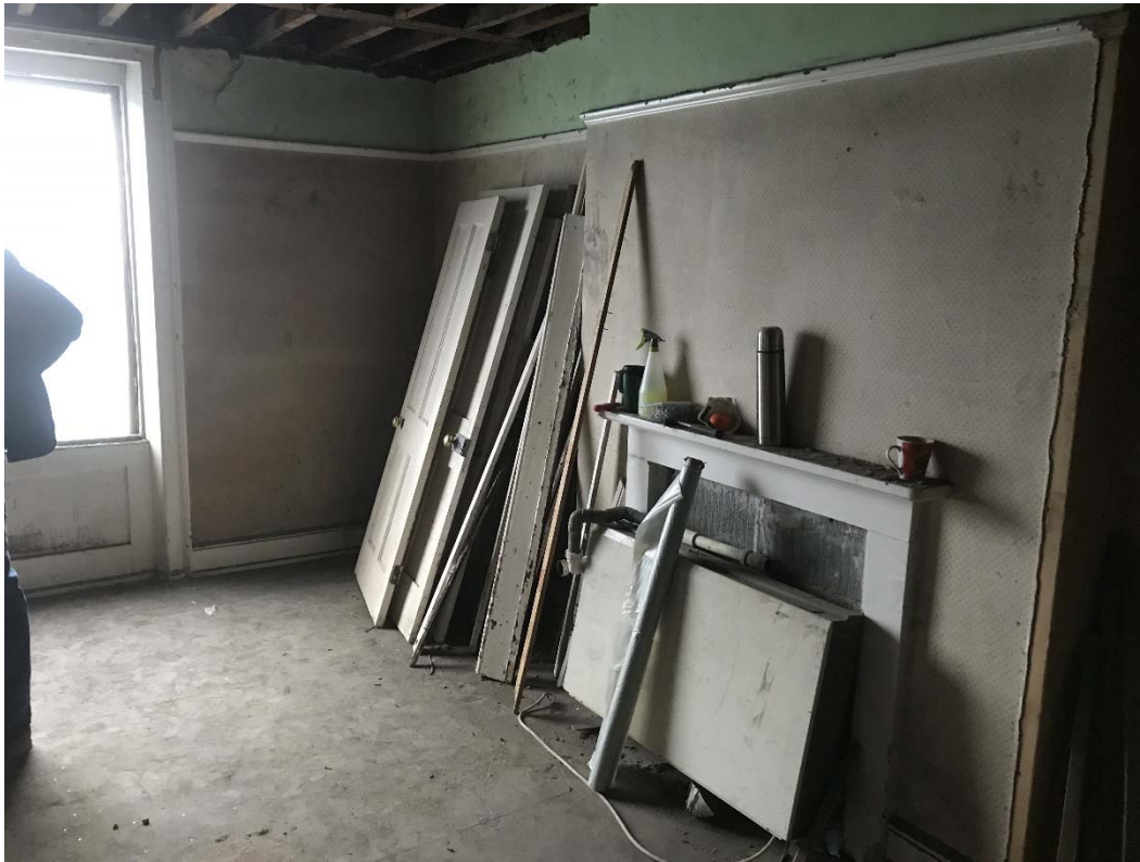
Fig 3 – Area of apartment generally unaffected, save the removed roof
