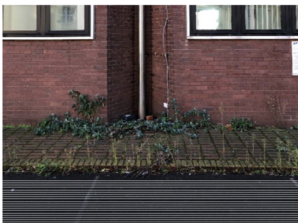
Figure 3 Emerging weeds in car park
