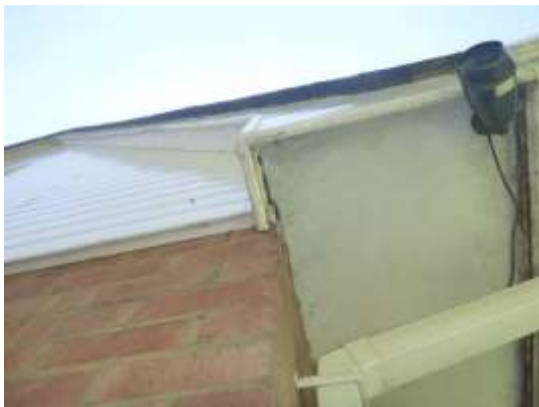
5. Cobwebbed gap under soffit at rear.
