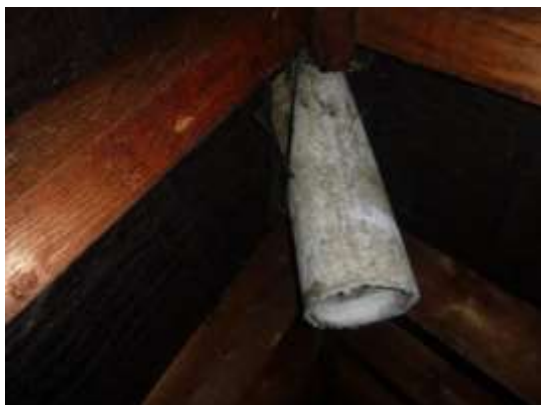
10. Roof vent allowing draught into roof space.
