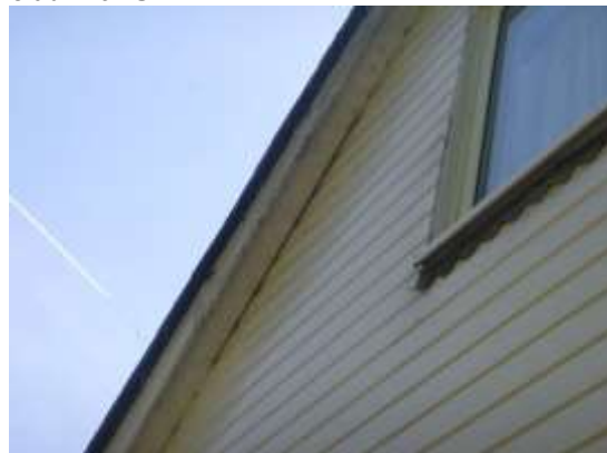
6. Cobwebbed barrow gap behind soffit at rear elevation unsuitable for bats.
