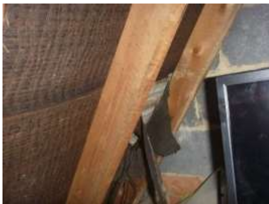
8. Tear in bitumen felt; tiles visible.
