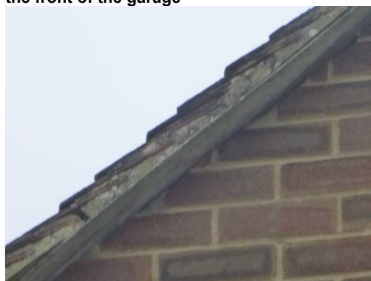
16. Gaps between the under-cloaking and bricks along the rear gable end of the garage
