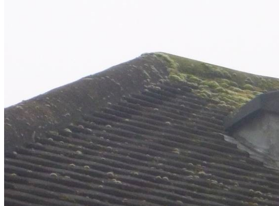
4. Occasional gaps under the roof tiles just below the hip tiles to the rear of the property
