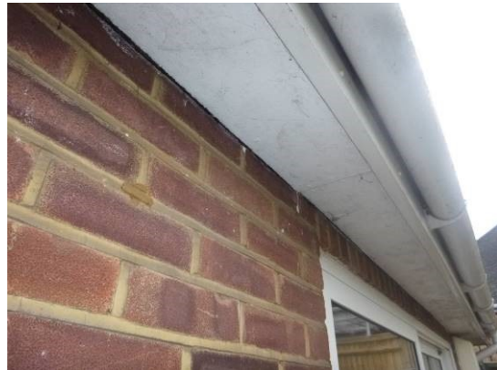
10. Gaps behind the soffits along the rear of the property
