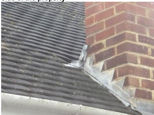
11. Gaps in tiles behind the chimney to the rear of the property
