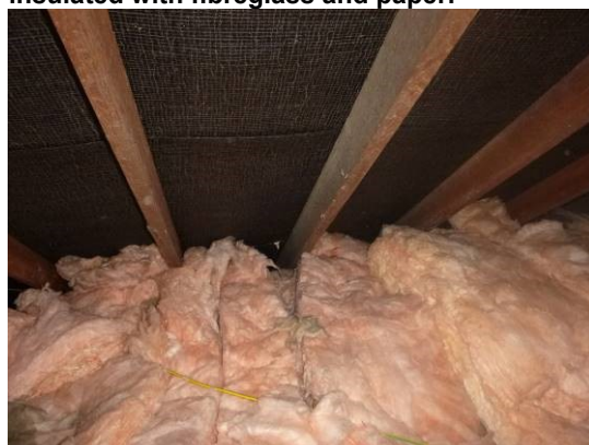
24. The eaves which were filled with fibreglass in places.
