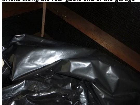
18. Internal view of the roof space with access blocked by a water tank
