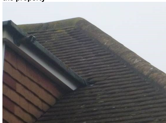
12. Potential gaps where the dormer window joined the main roof
