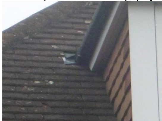
6. Broken roof tile to the front of the property
