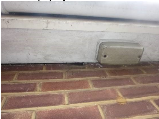
9. Gaps behind the soffits along the eastern side of the property
