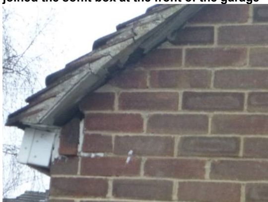
17. Crack in the mortar and a large gap where the under-cloaking was damaged on the rear gable end of the garage
