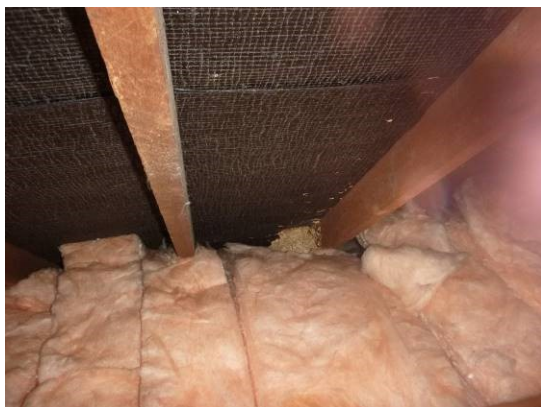
25. Wasps' nest present along the rear (north facing) side of the eaves space
