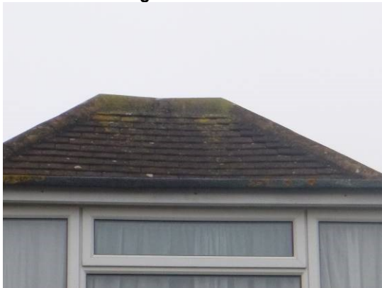
5. Lifted roof tiles just below the ridge to the front of the property and just below the hips
