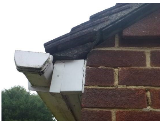
15. Large gap present where the verge tiles joined the soffit box at the front of the garage
