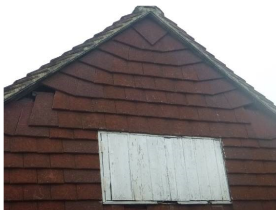
14. Hanging tiles missing on the gable end to the front of the garage
