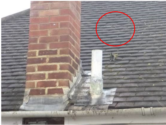
7. Sunken roof tiles behind the chimney on the rear of the property
