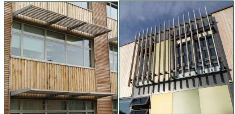
Figure 7. External solar shading 2
