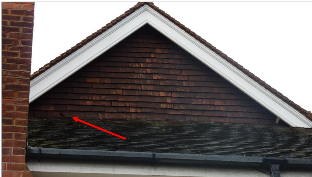
Photograph 6: Tightly fitted hanging tiles with one broken hanging tile on lowest course
