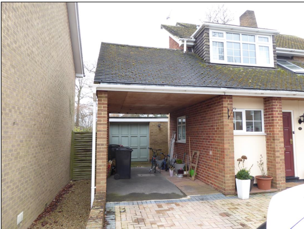
Figure 6. Roof over car port, 11 Yarnton Close, Emmer Green. 13.03.18
