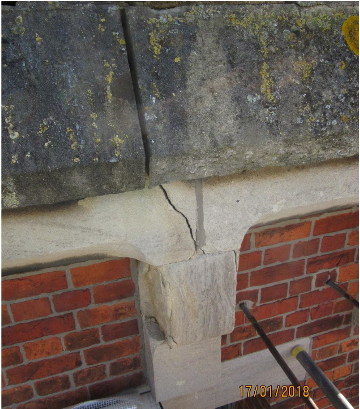
Photograph 6 - Cracking to bathstone corbel beneath turret parapet and delamination of corbel side
