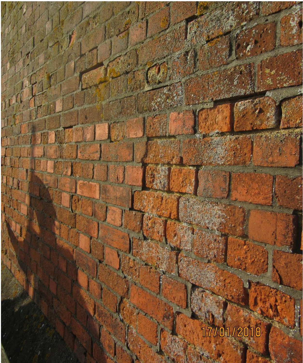
Photograph 1 - Brickwork erosion from cement mortar works
