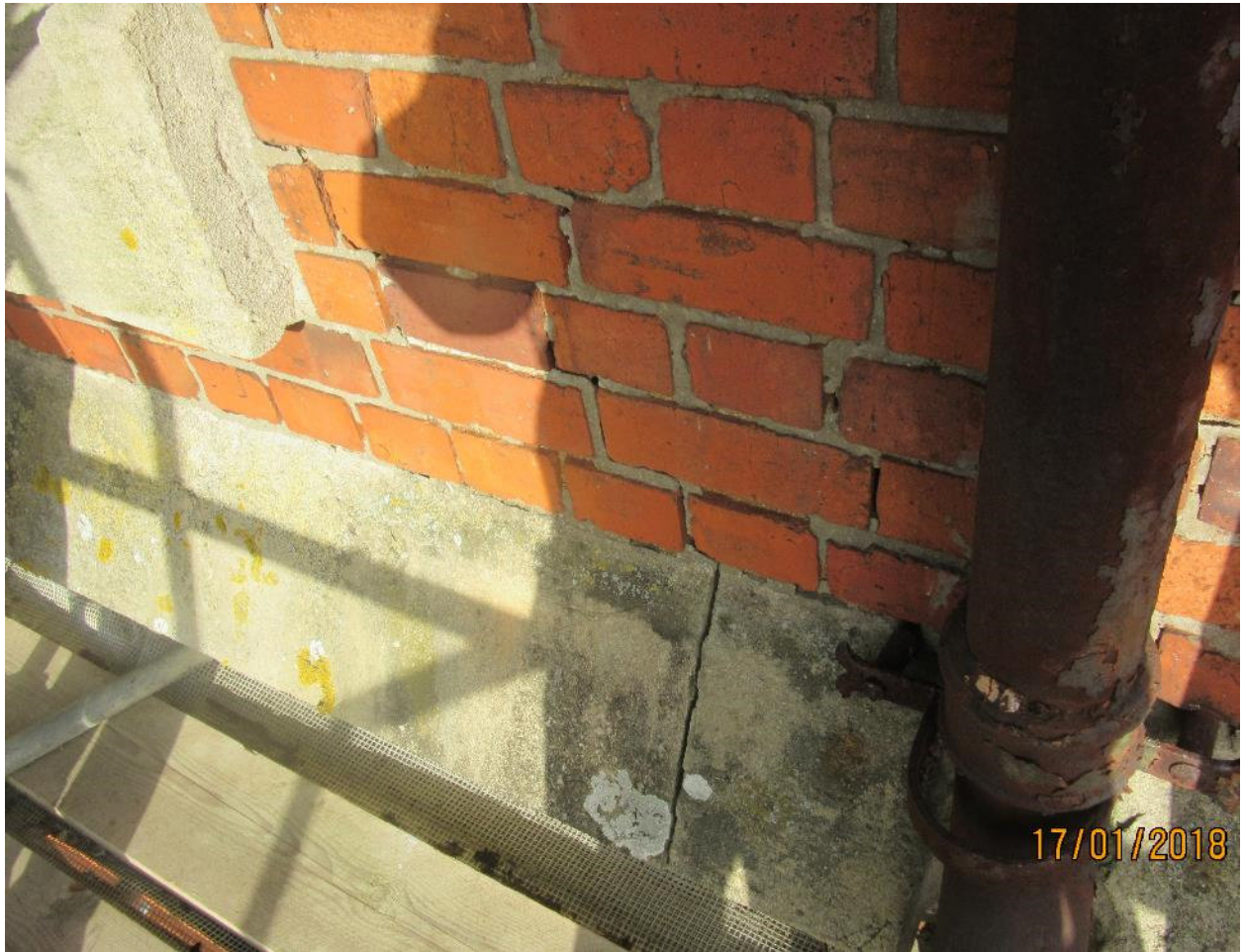
Photograph 4 - Cracking to parapet walls
