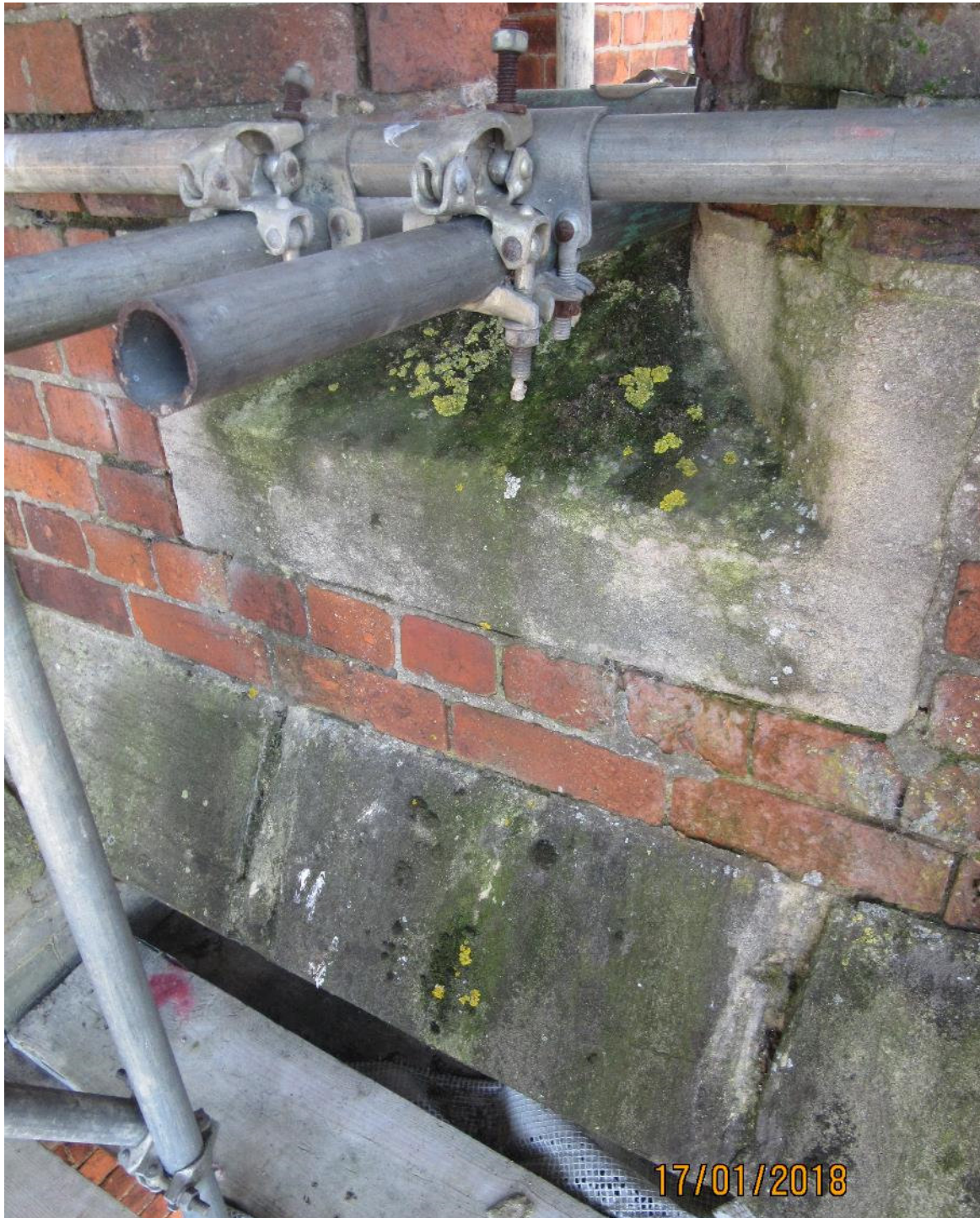
Photograph 2 - Bathstone eroded beneath castellation
