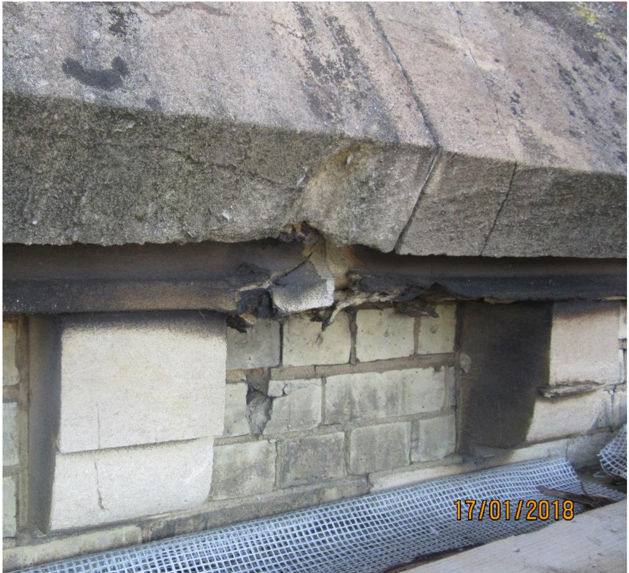
Photograph 3 - Under side of bathstone delaminating beneath eroded cracked area
