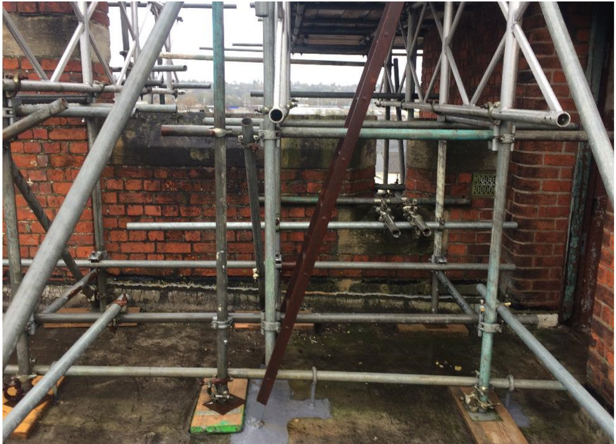
Photograph 11 - Scaffold eye bolts penetrating the roof finish
