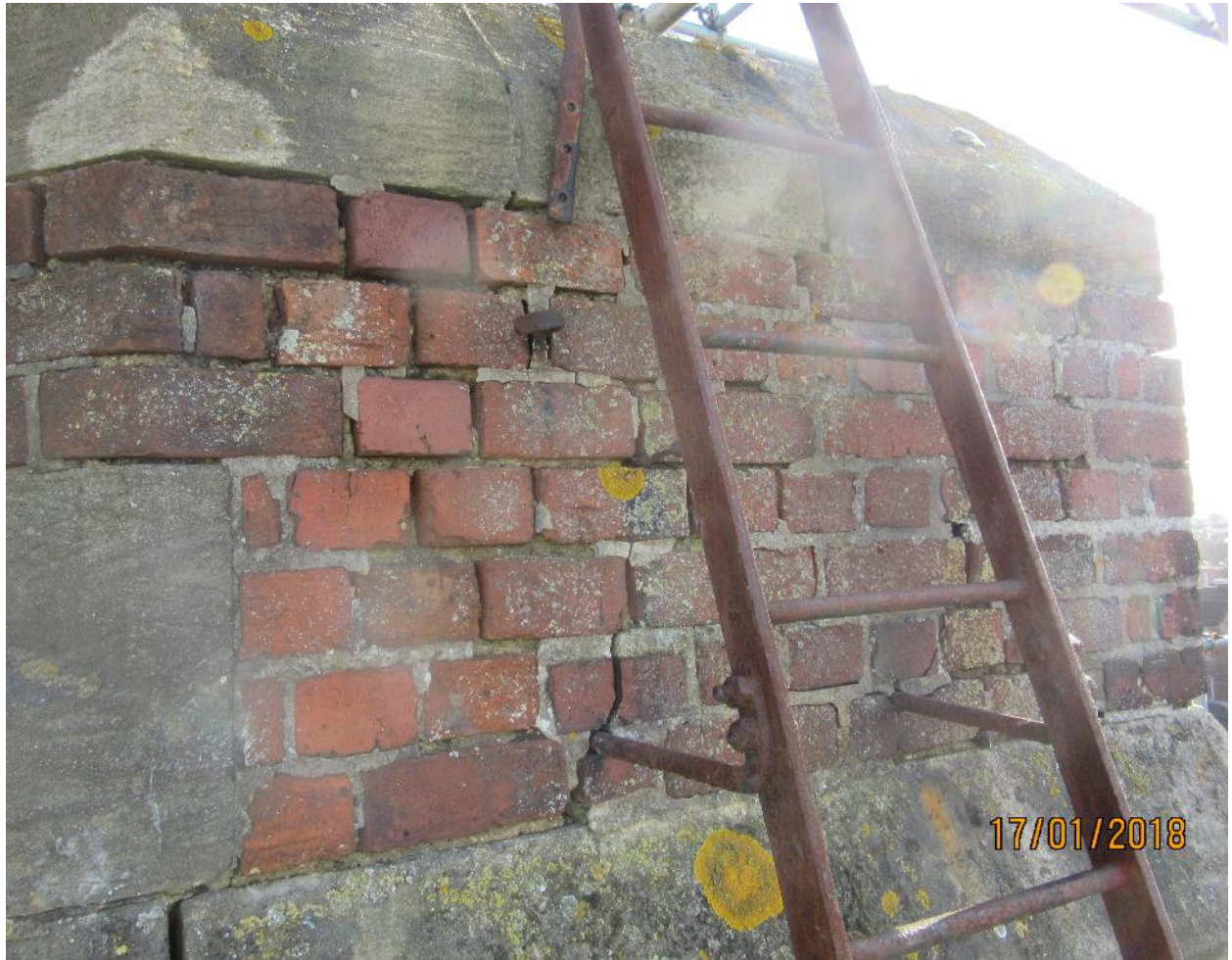
Photograph 5 - Cracking to brickwork turret at ladder fixings
