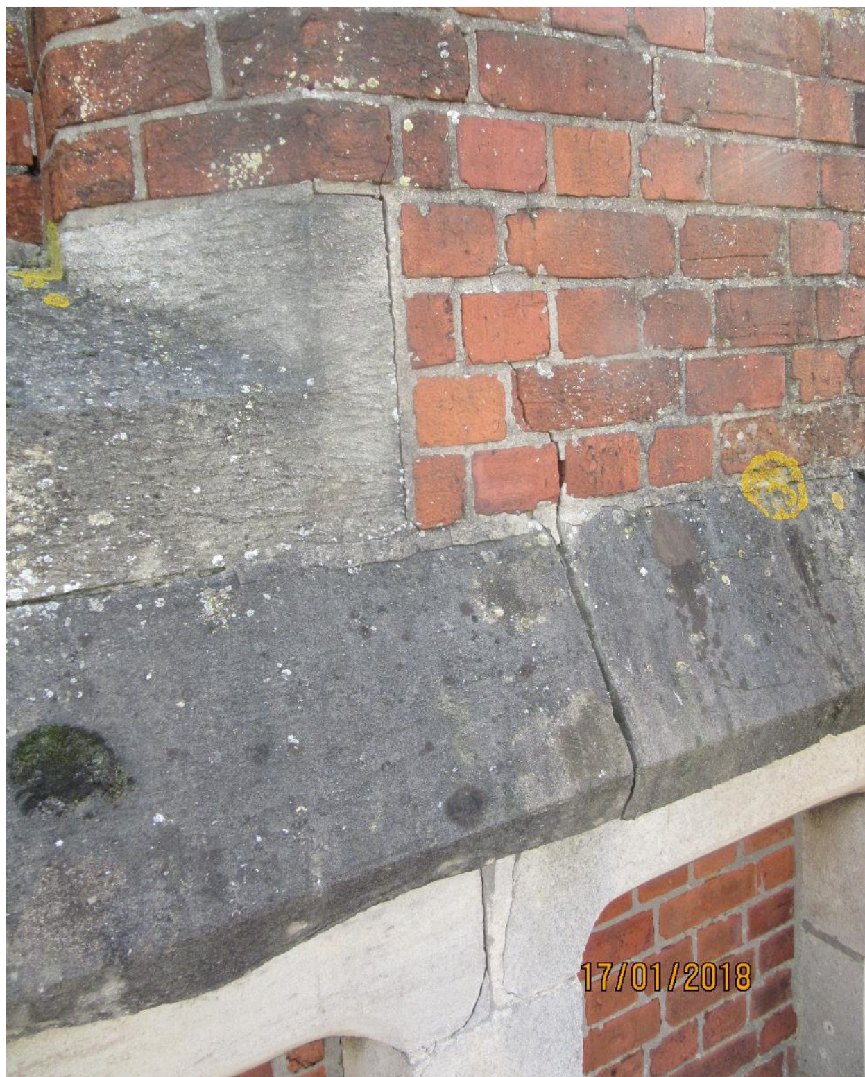
Photograph 7 - Cracking to bathstone corbel beneath turret parapet
