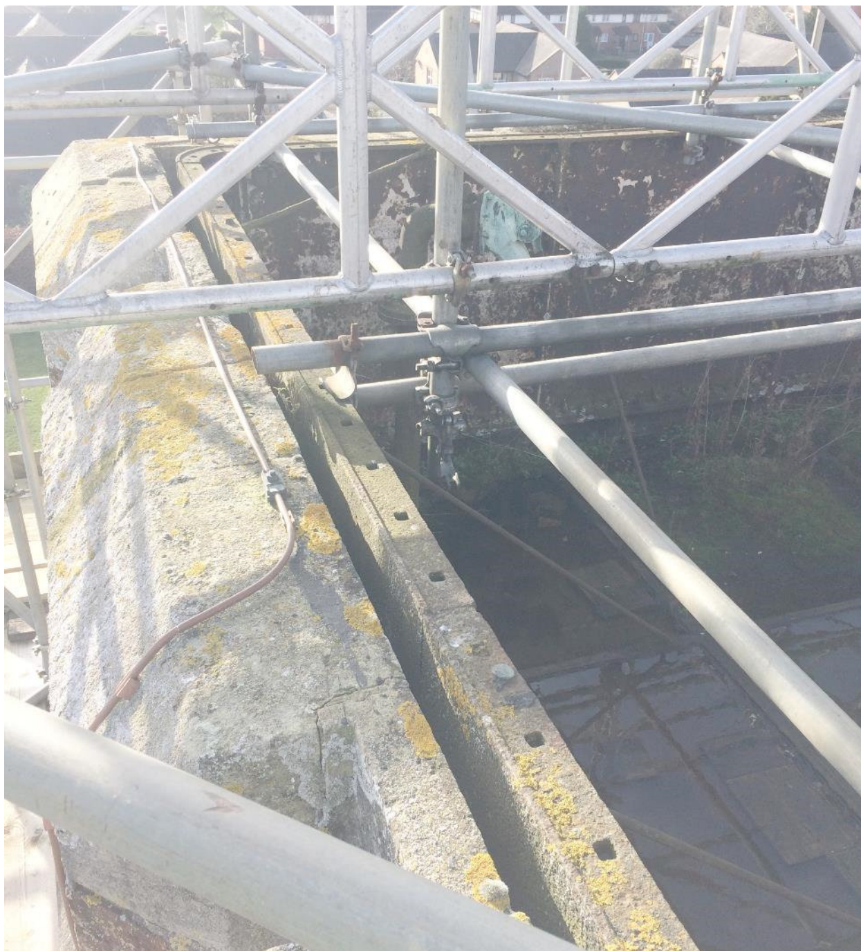
Photograph 9 - Gap between water tank and parapet
