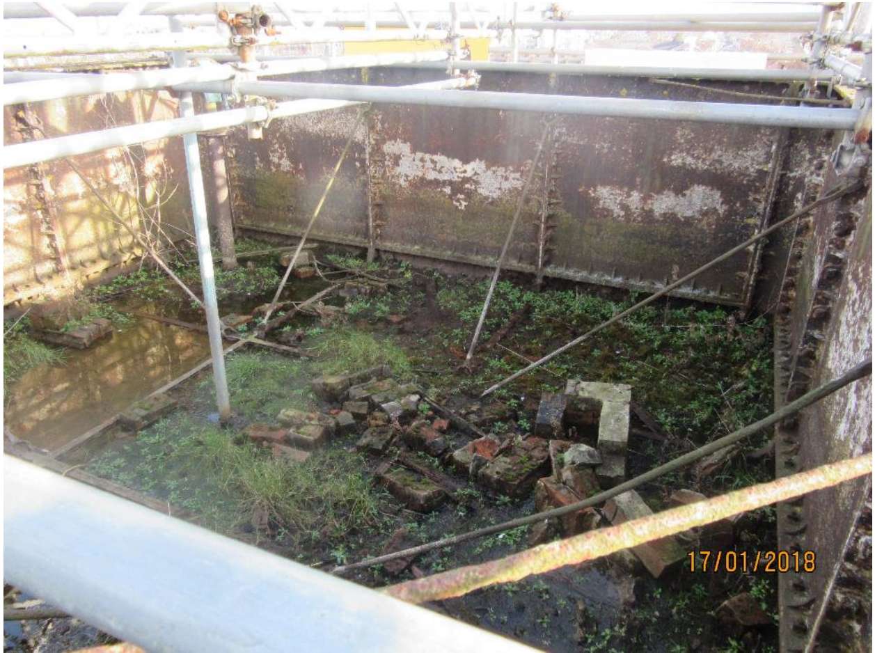
Photograph 10 - Collapsed chimney stack within water tank
