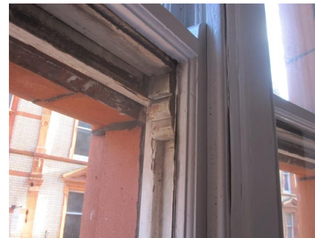
Rot on front sash windows
