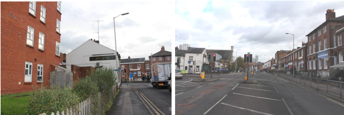
Figure 3 - Existing street lighting around the junction of Bedford Road (left) and Oxford Road (right).
