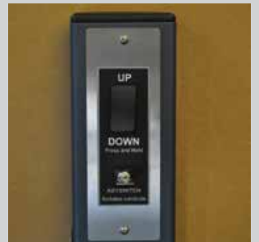
Key Switched Controls
