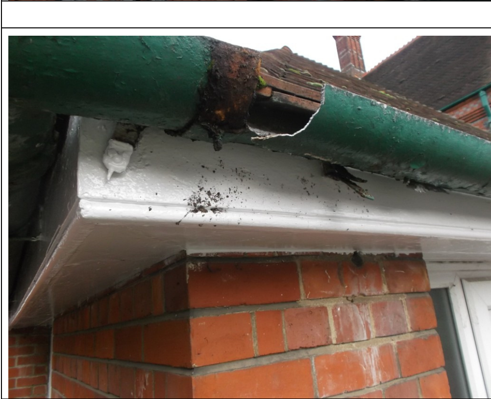
10) East Wing, Rear Elevation Single-Storey Addition. Broken cast iron gutter.
