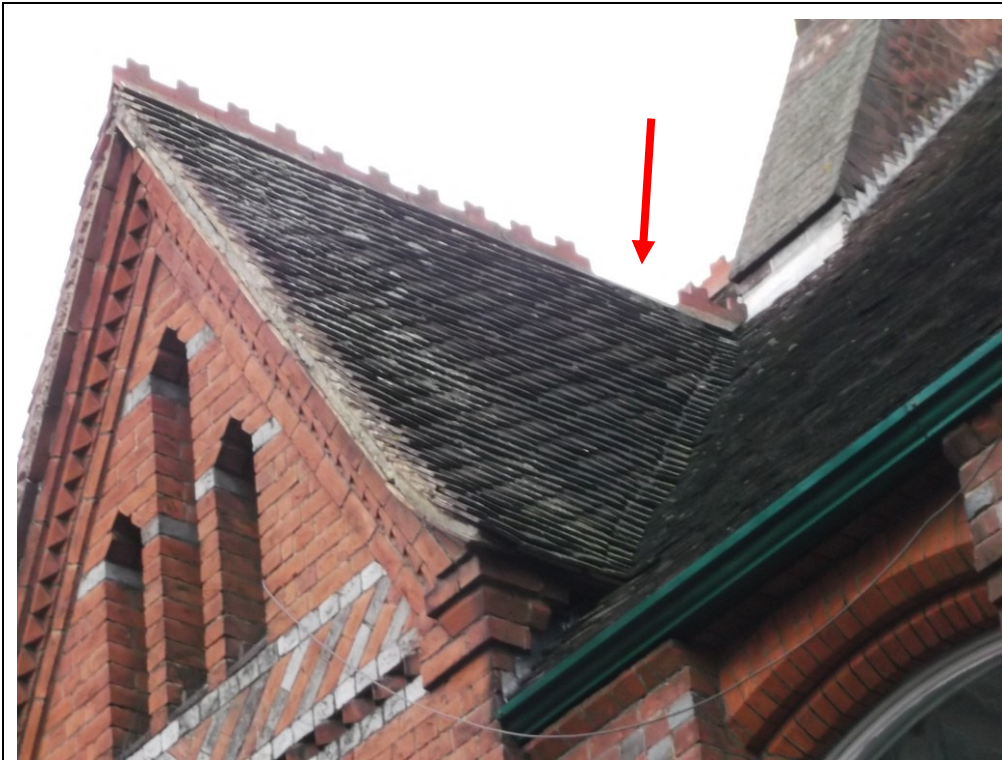
9) East Wing, Rear Elevation. Note missing ridge tile to dormer roof.
