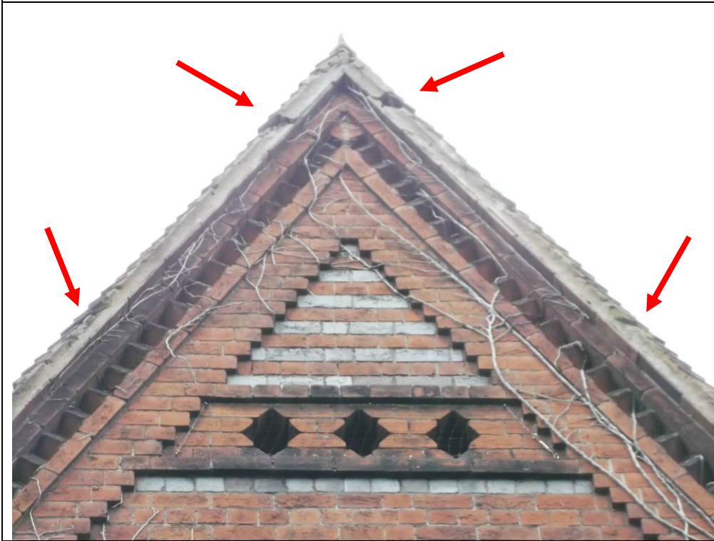
18) East Wing, East End Elevation. Note erosion to verge pointing.
