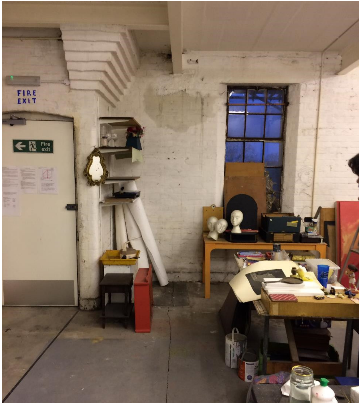
Photograph 17 - Damp brickwork beneath beam bearing on East elevation, 3 rd floor
