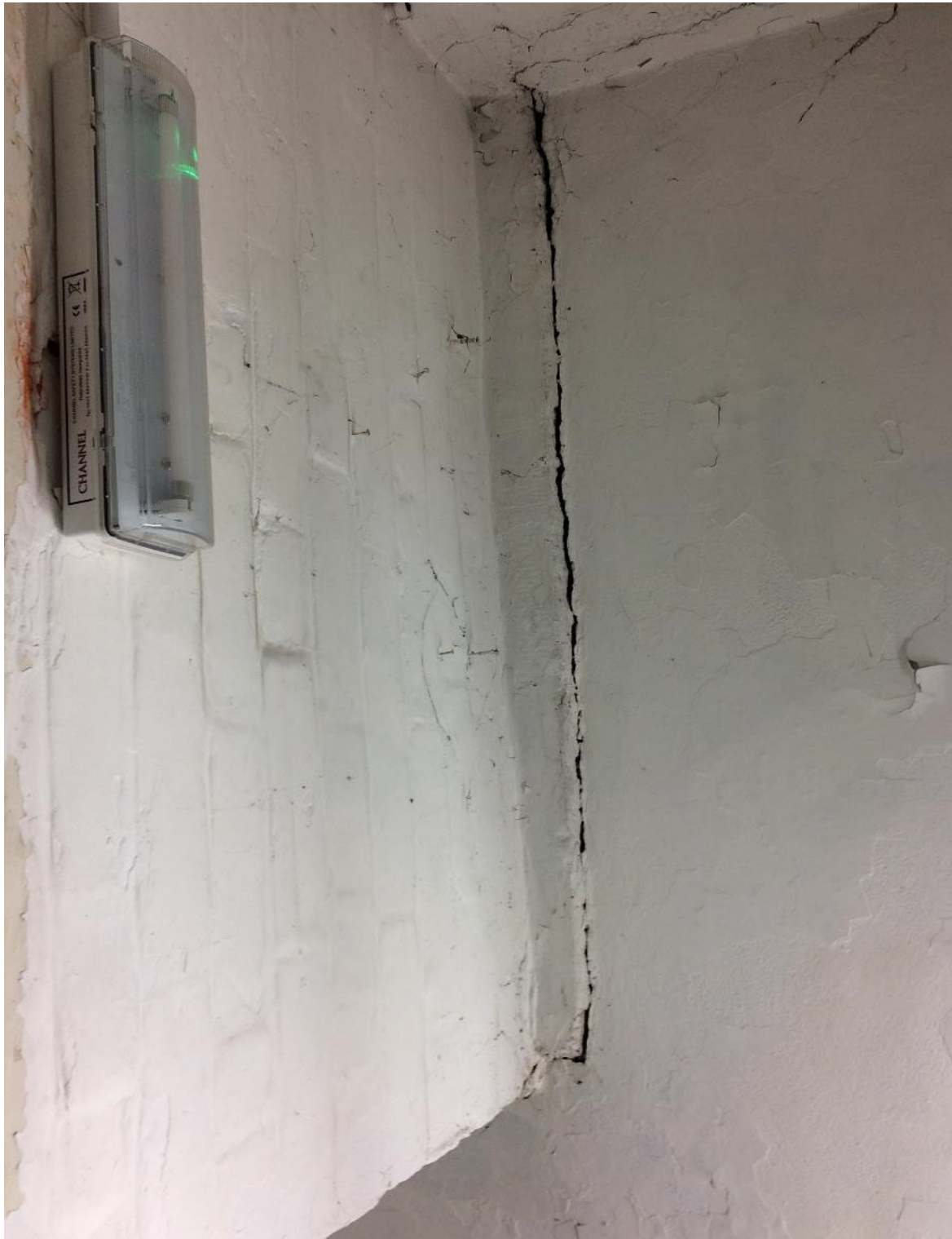
Photograph 18 - Crack to underside of 3 rd floor slab, above doorway to the North East tower
