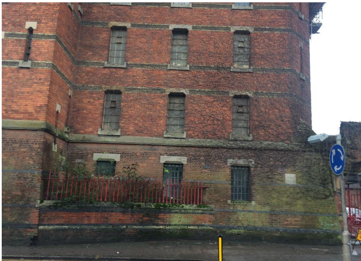
Photograph 23 - Damp external wall below first floor
