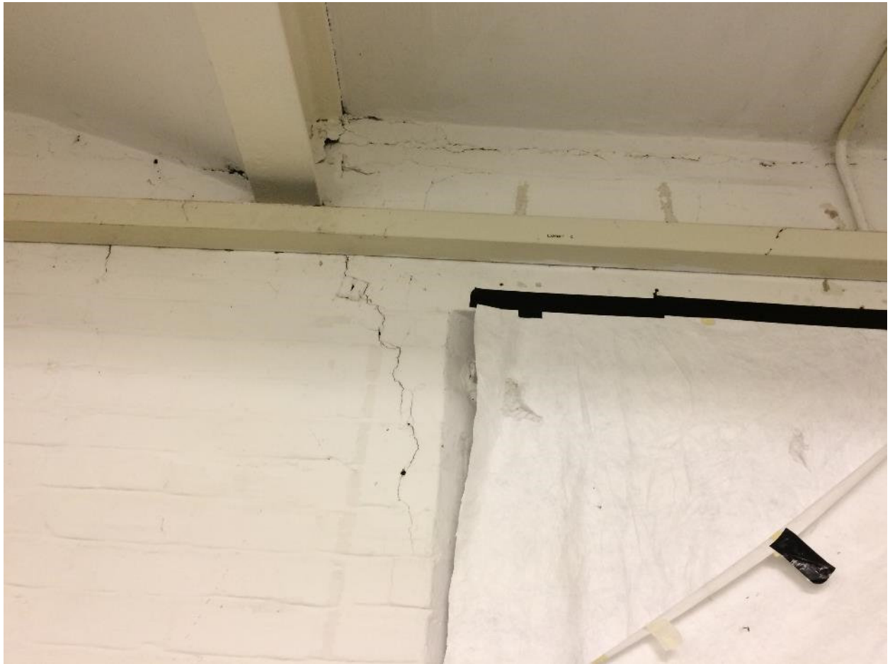
Photograph 22 - Cracking to walls beneath beam bearing
