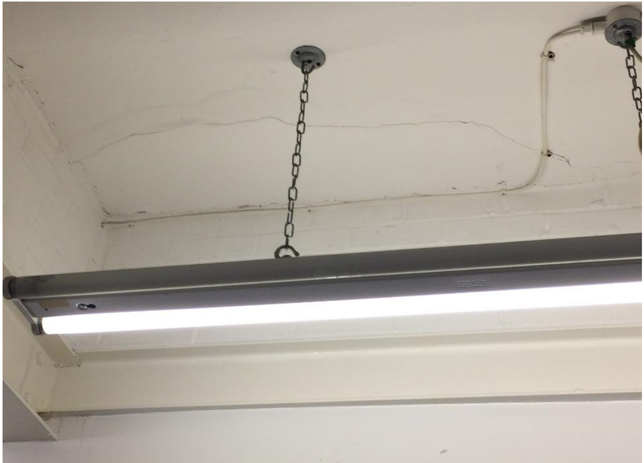
Photograph 15 - Cracking to underside of barrel vaulted roof slab
