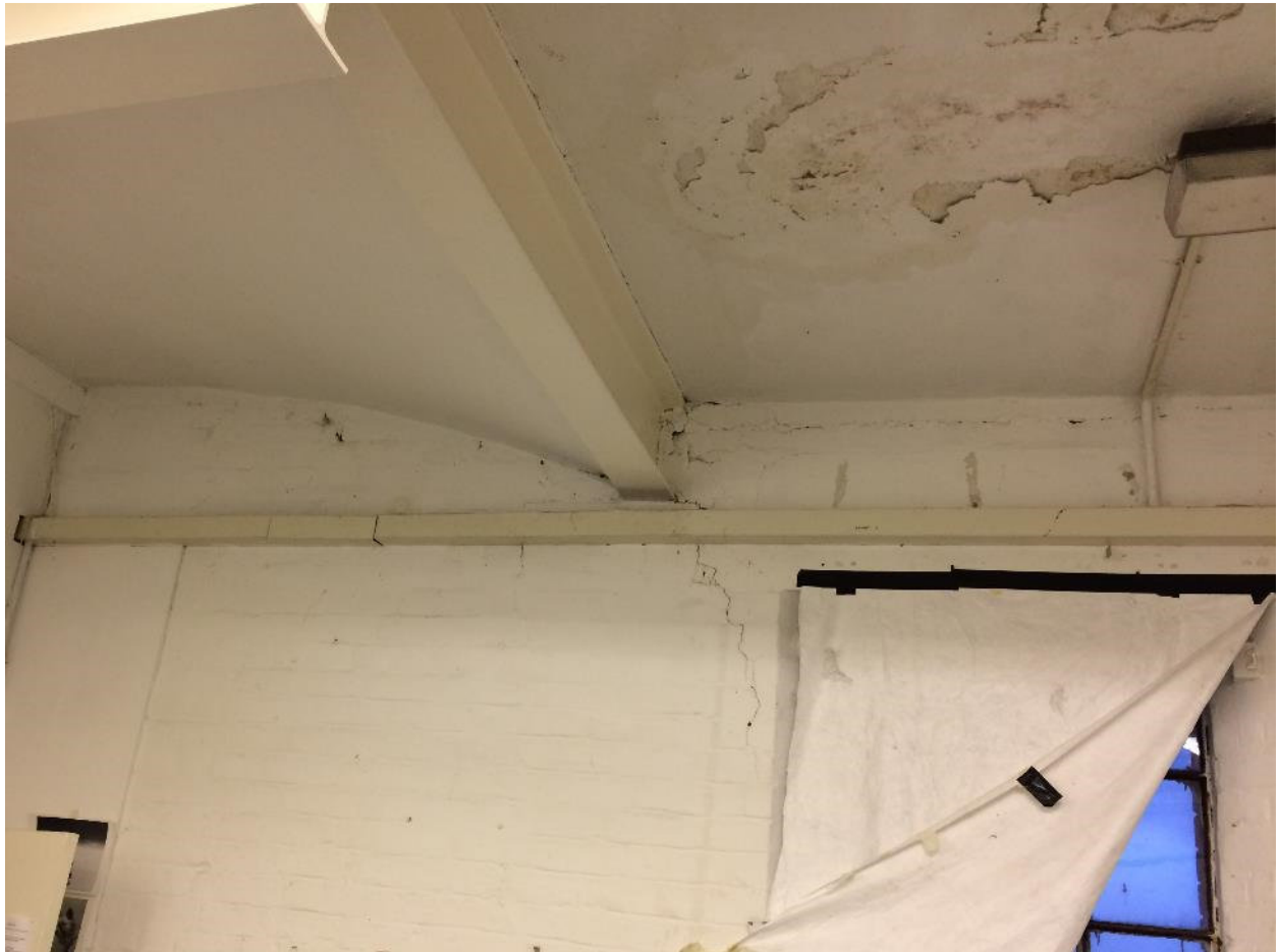
Photograph 13 - Damp marks and deterioration of ceiling finish below eye bolts SW turret
