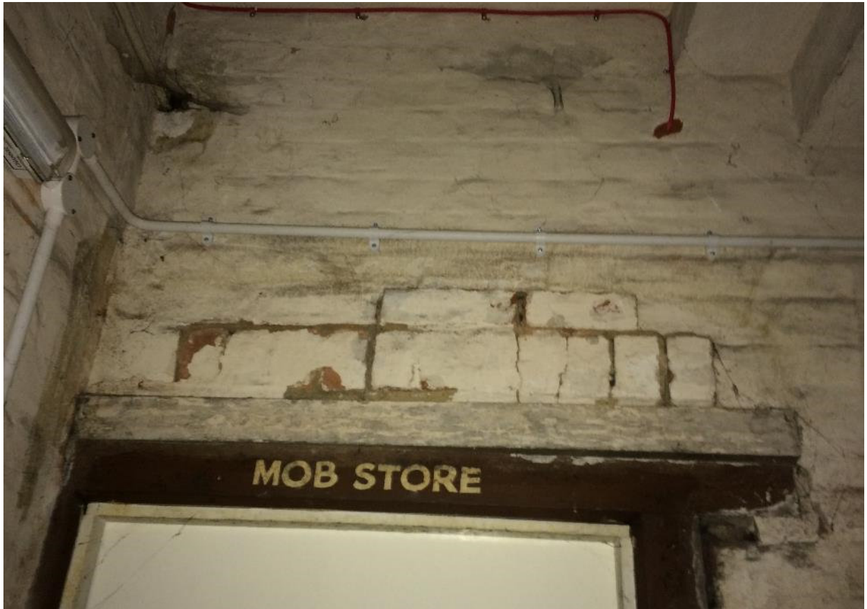
Photograph 25 - Brick dislodged over door lintel from NE tower
