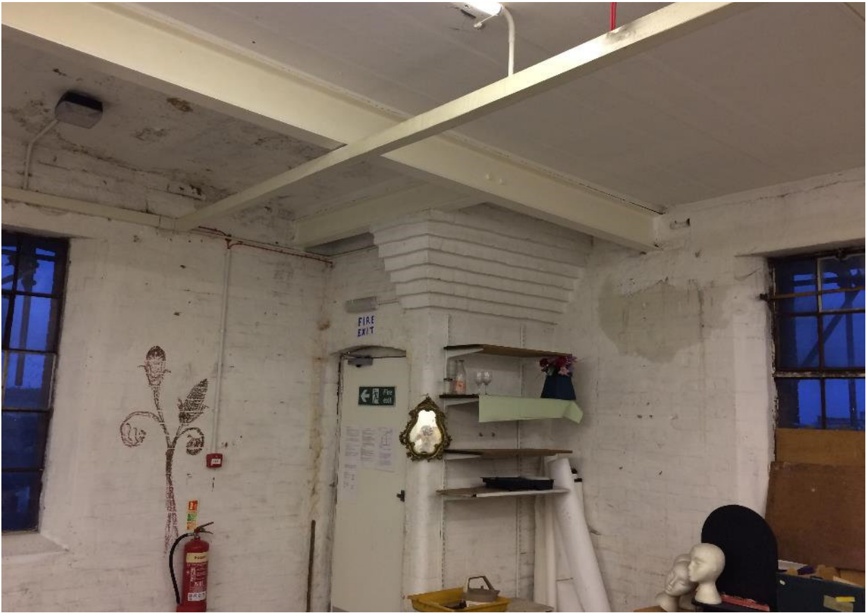
Photograph 12 - Damp marks and deterioration of ceiling finish below eye bolts NE turret
