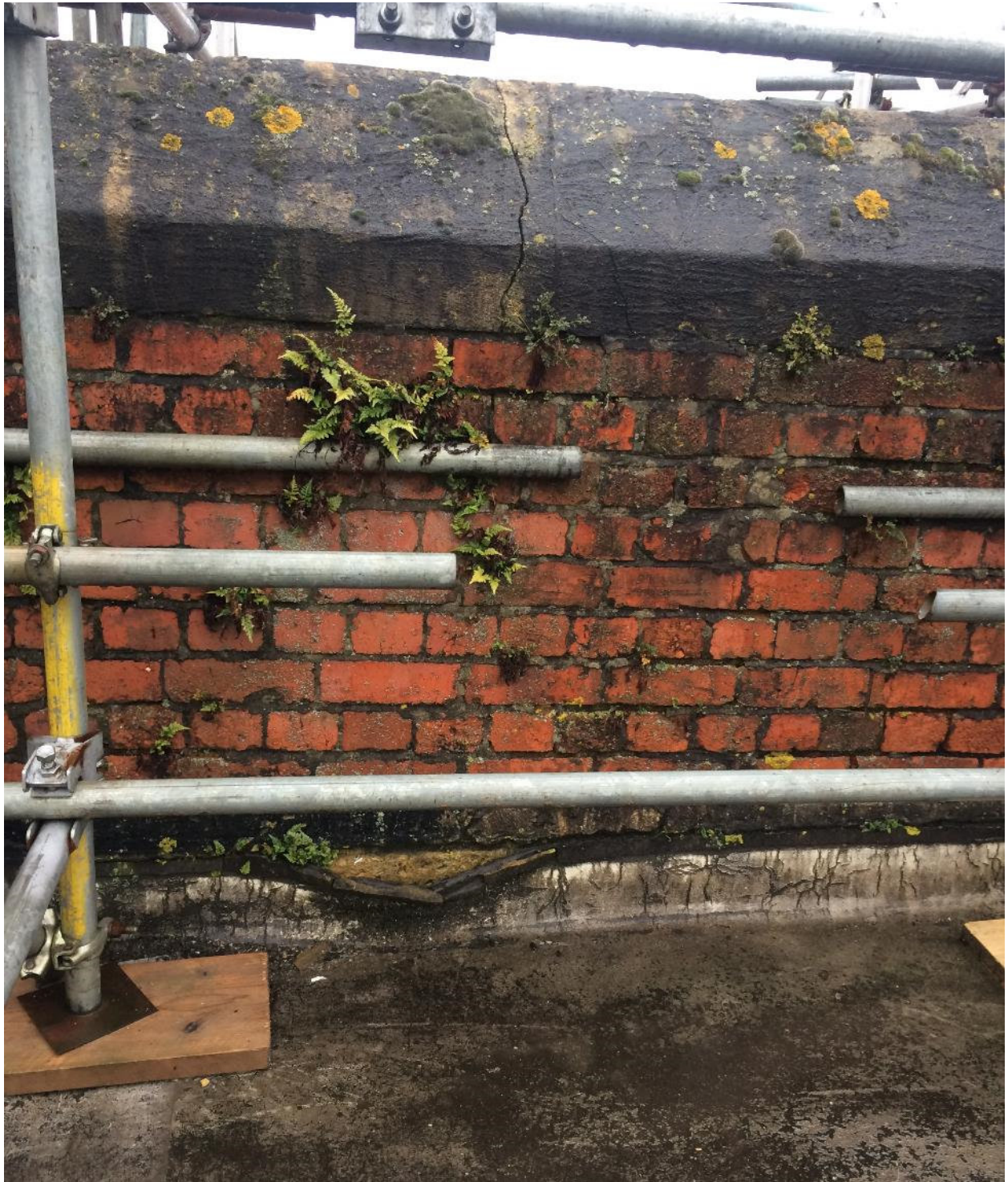
Photograph 14 - Asphalt upstand detached from wall, exposing bath stone
