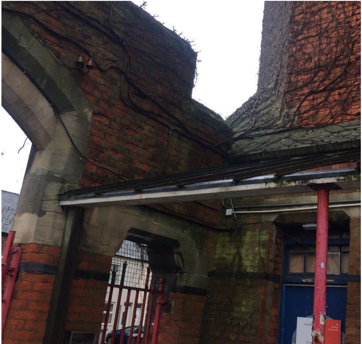
Photograph 26 - Timber post supporting the veranda is damp.
