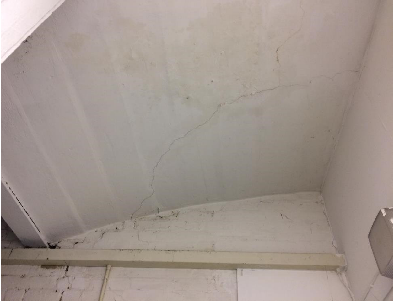
Photograph 16 - Cracking to underside of barrel vaulted roof slab
