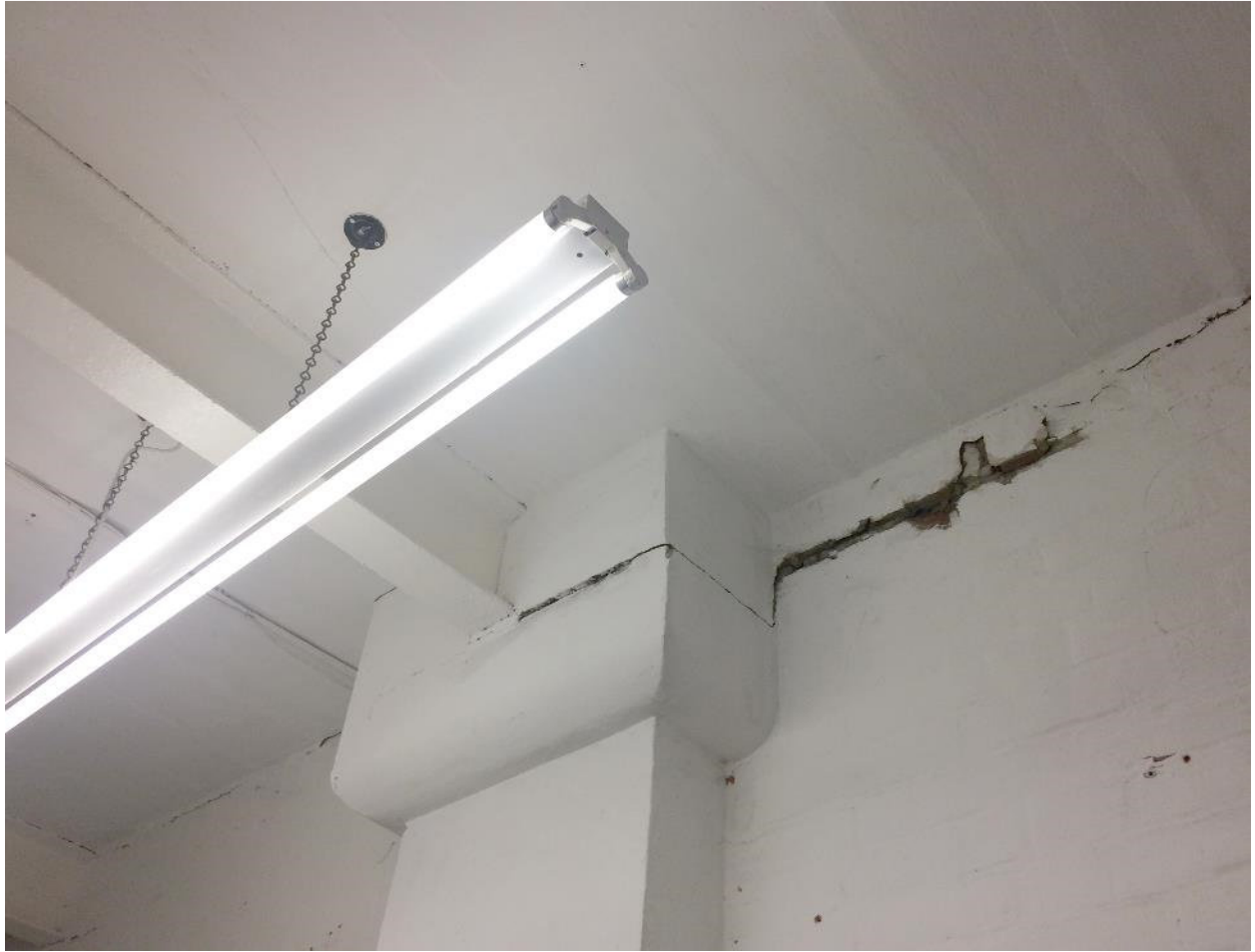
Photograph 21 - Cracking to the stone capital around the beam bearing
