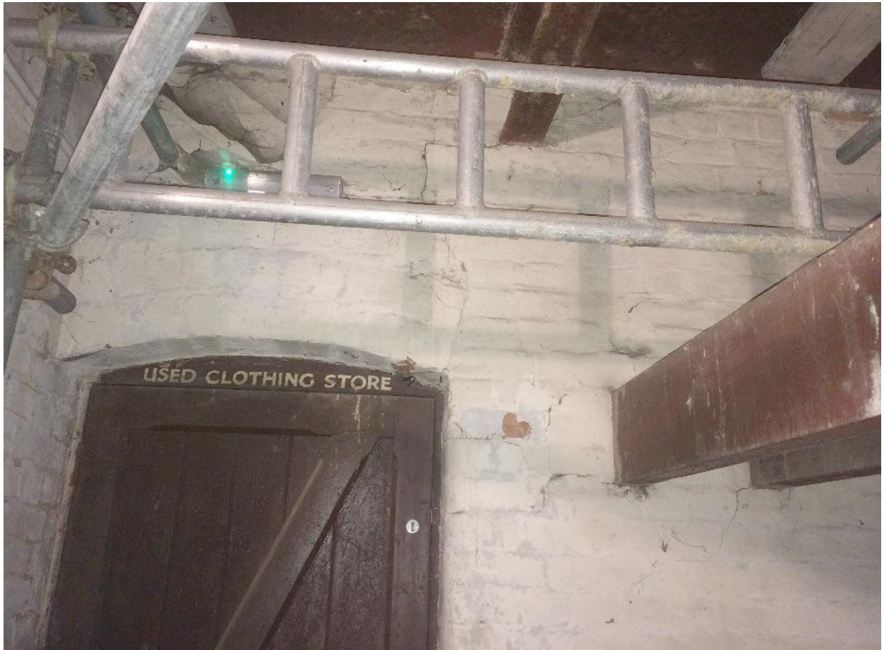
Photograph 24 - Cracking to tower wall beneath water tank beam
