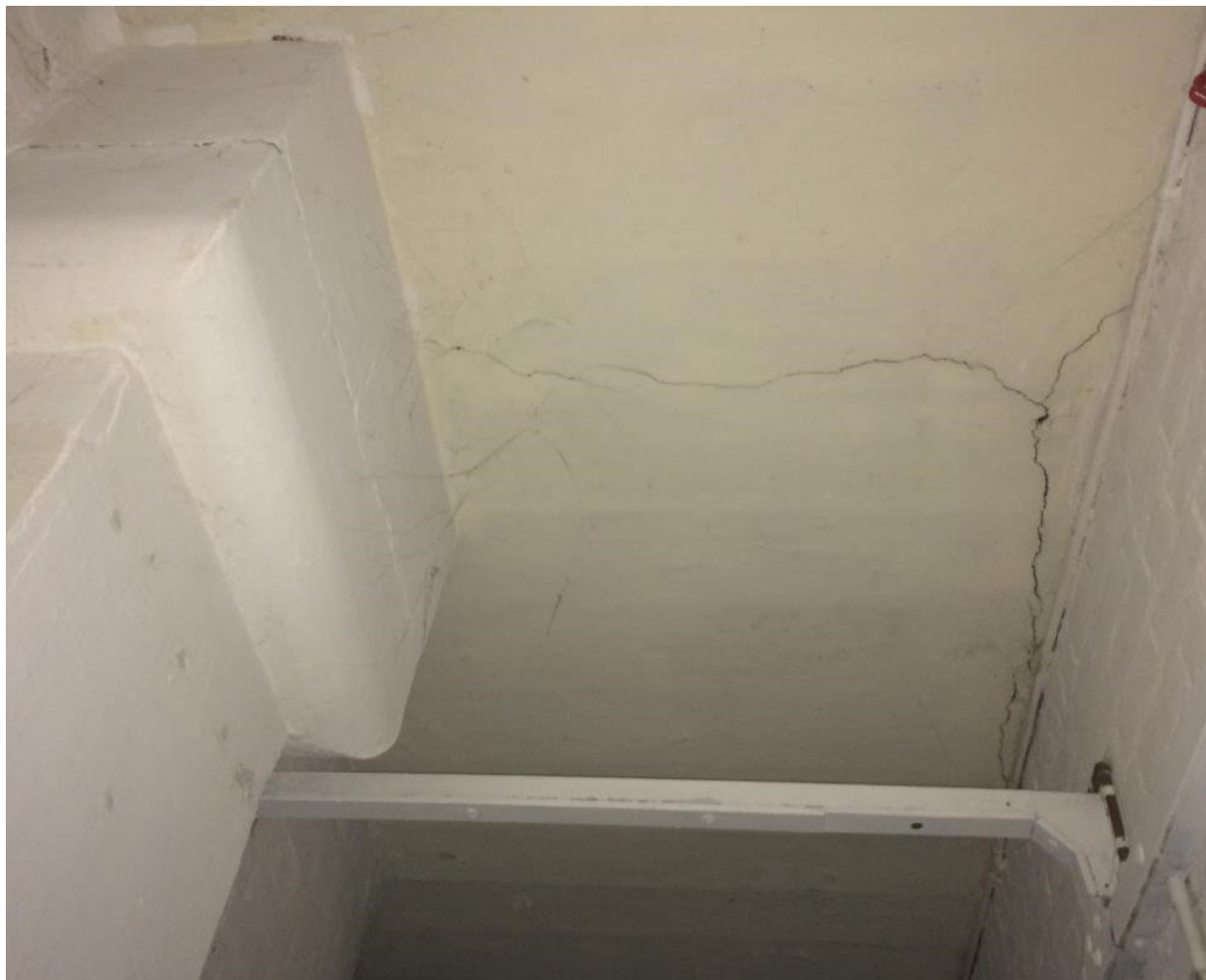
Photograph 20 - Cracking to the underside of the First-floor slab
