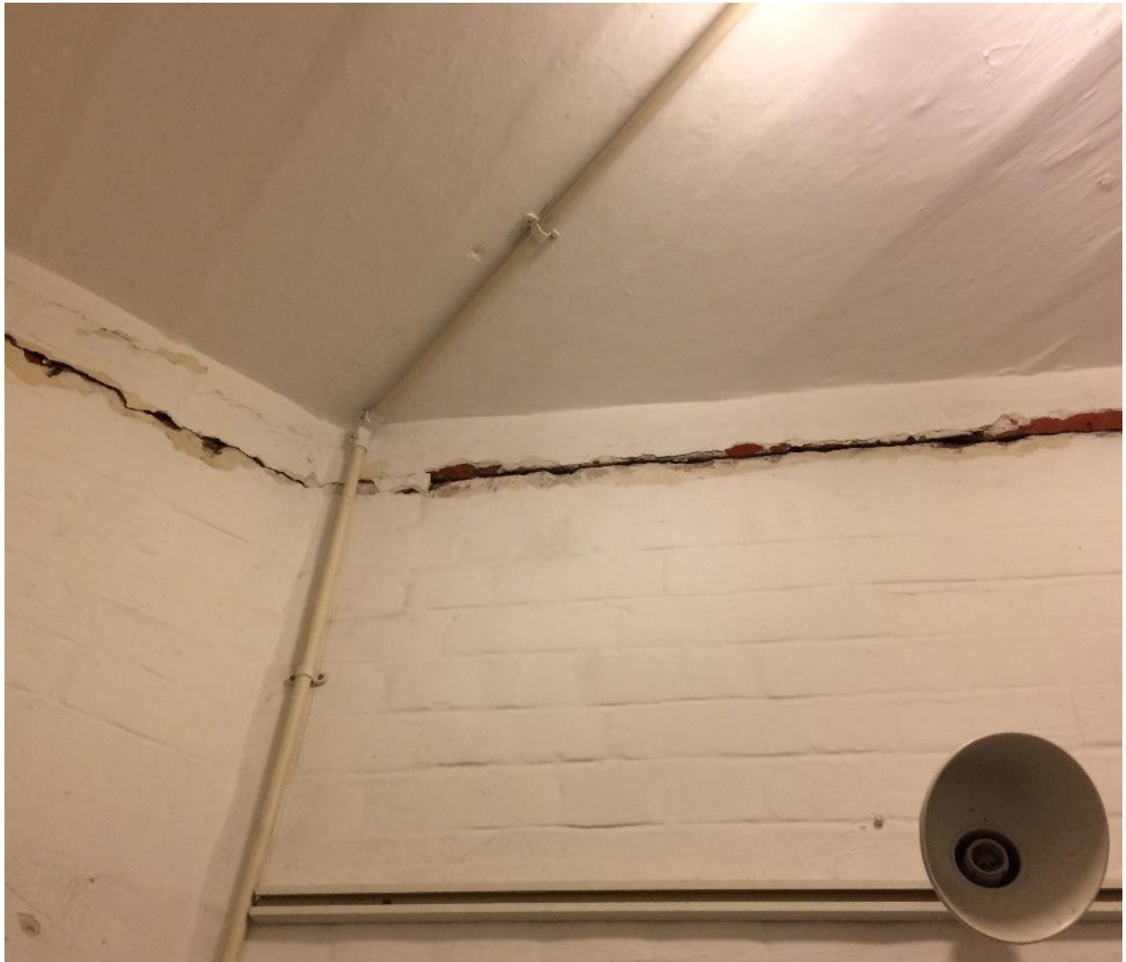
Photograph 19 - Crack to bed joint beneath 2 nd floor slab over NW chamfered corner
