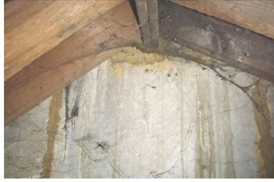
16. The cobwebbed gable end.
