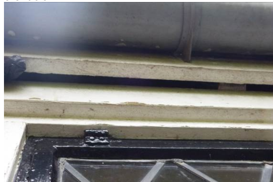
6. The gap behind the barge board on the front elevation.
