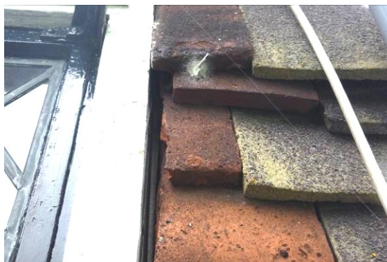
8. The gaps between the hanging tiles.
