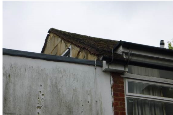
4. The lifted verge tiles visible on the rear elevation
