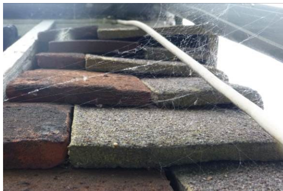
10. The gaps behind the corner hanging tiles.
