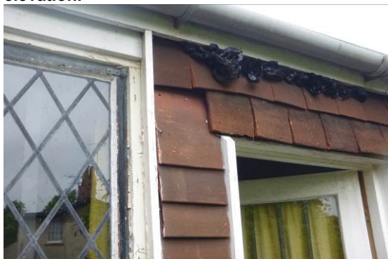
9. The gaps into the eaves above the hanging tiles and the missing hanging tile.
