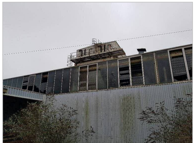
LAUNDRY BUILDING (NOTE: WATER TANK IS LIKELY TO HOLD STAGNANT WATER, RISK OF LEGIONELLA / LEPTOSPIROSIS ETC.)
