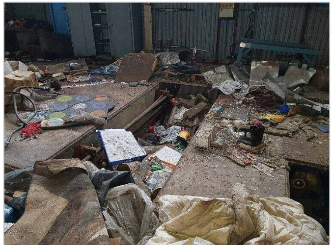
VOIDS IN FLOORS WITHIN INCINERATOR BUILDING (NOTE: THESE ARE NUMEROUS THROUGHOUT, SOME CONTAINING FAECES, NEEDLES/SYRINGES & STAGNANT WATER)
