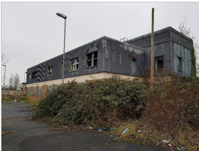
PORTMAN HOUSE (NOTE: EXTENSIVE FIRE DAMAGE)
