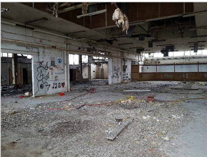
VIEW INSIDE LAUNDRY BUILDING (NOTE: EXTENSIVE FIRE DAMAGE, COLLAPSED ASBESTOS CEILINGS, ASBESTOS FRAGMENTS SCATTERED ACROSS GROUND)
