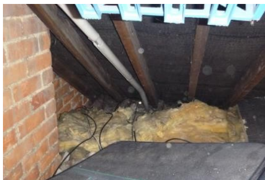
14. Hole at eaves at front of house where cables were running through.
