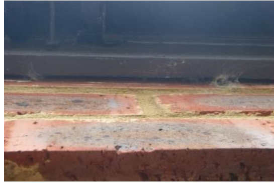
8. Cobwebbed gap behind bargeboard of rear extension.
