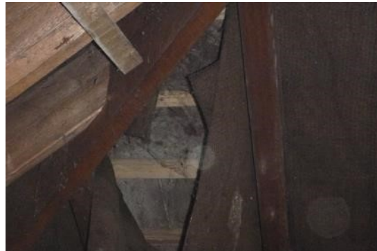
12. Tear in felt exposing tiles underneath at rear of house.
