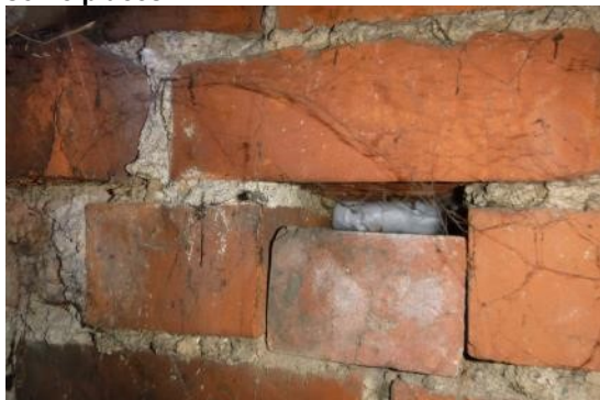
15. Gap in brickwork of internal gable.
