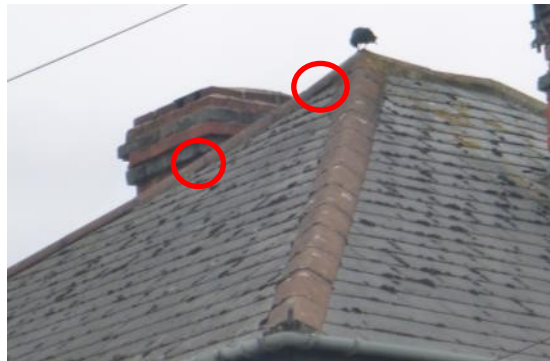
6. Two gaps underneath hip tiles on the northern roof elevation.
