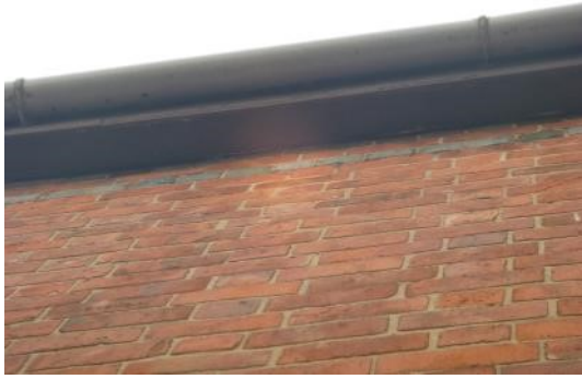
7. Tightly sealed soffit at the side of the house.
