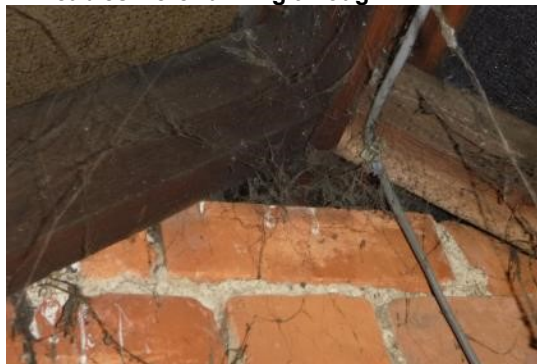
16. Heavily cobwebbed gap at apex of internal gable.
