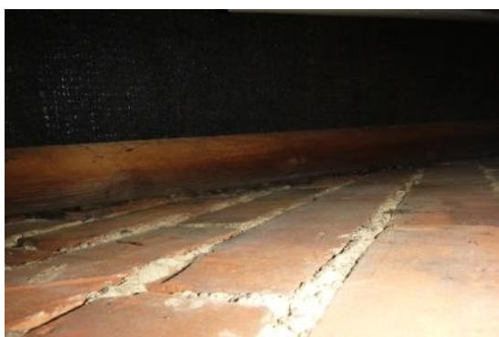
17. Cobwebbed gap between rafters and brickwork of chimney.
