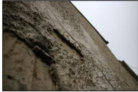
Photo 54: building 203 damaged pebble dashing
