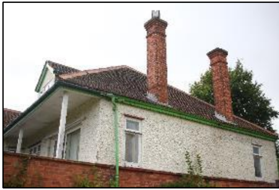
Photo 43: Building 201 slipped tiles
