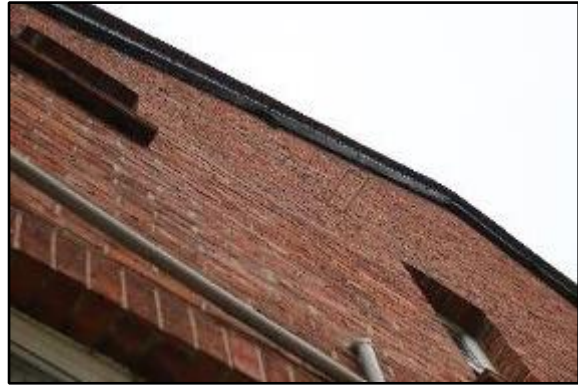
Photo 33: building 199 gaps in soffits
