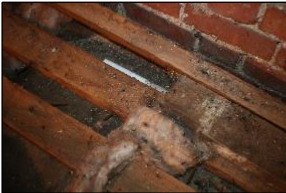
Photo 36: building 199 bat droppings
