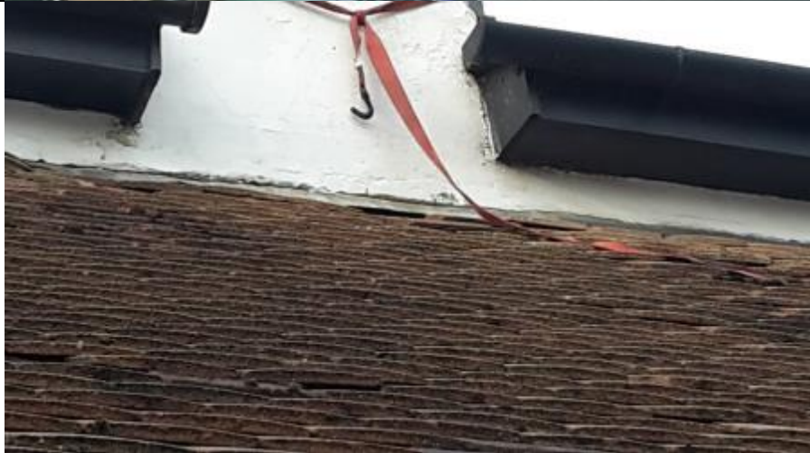
Photo 3: missing tile under lead flashing on the side of the garage roof.
