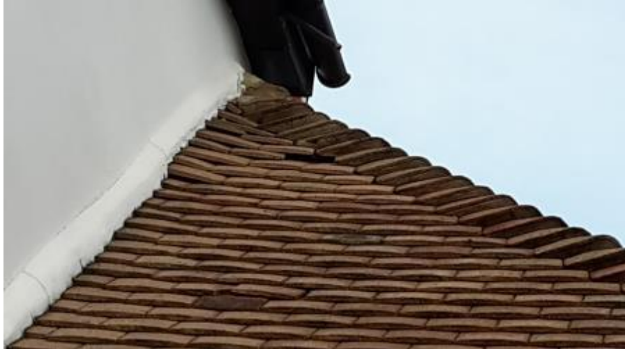
Photo 4: missing tile on the front of the garage roof.
