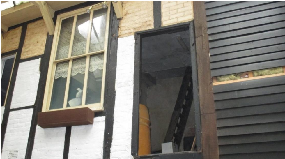
Figure 5.53 – A space to the back of the rear range is sealed off at first floor level, and only accessible via a step ladder from the second floor
