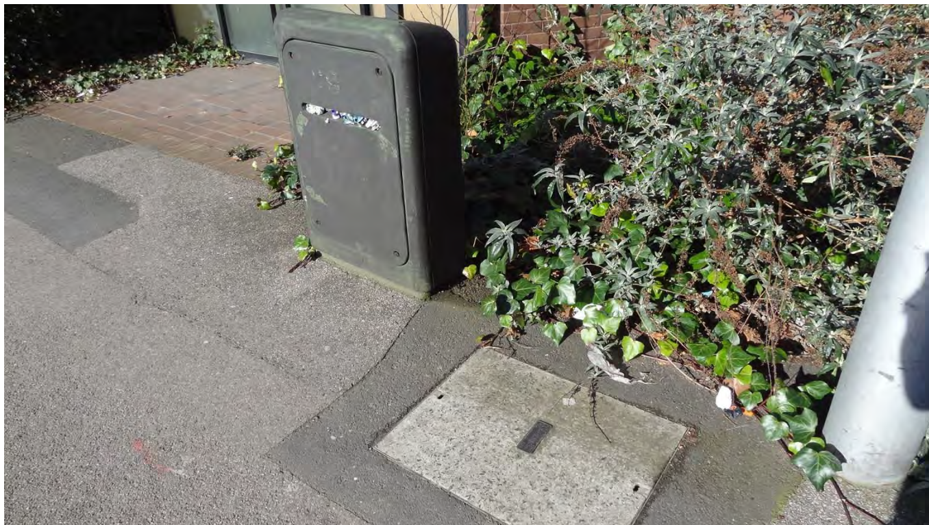
Figure 7 – Cabinet in Queens Road adjacent to Clarendon House
