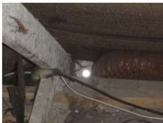
12. Hole in soffit; daylight visible.
