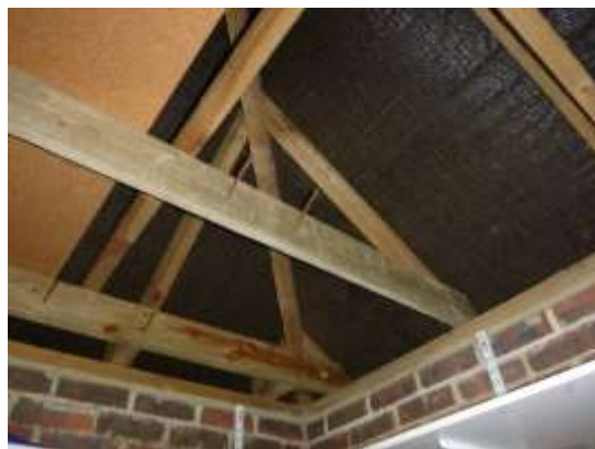
14. Garage lined with bitumen and ground floor open to roof void.
