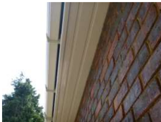
8. UPVC soffits on garage tight to brickwork.
