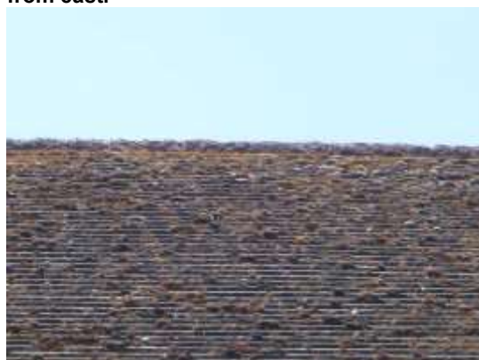
4. Tiles at rear covered in moss and fitted tightly.
