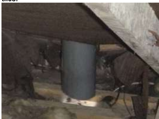
11. Tear in felt around pipe.
