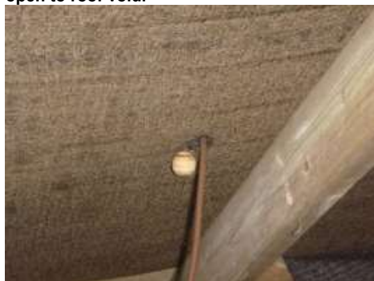
16. Small wasps' nest in south-western side of roof.
