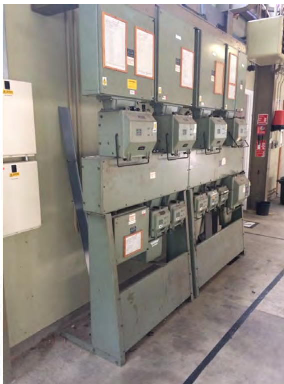
Photo 3 – Redundant fuse board in Engineering building. No transformer was noted in the accessible parts of the building. Site management confirms no transformer was present in the building.
