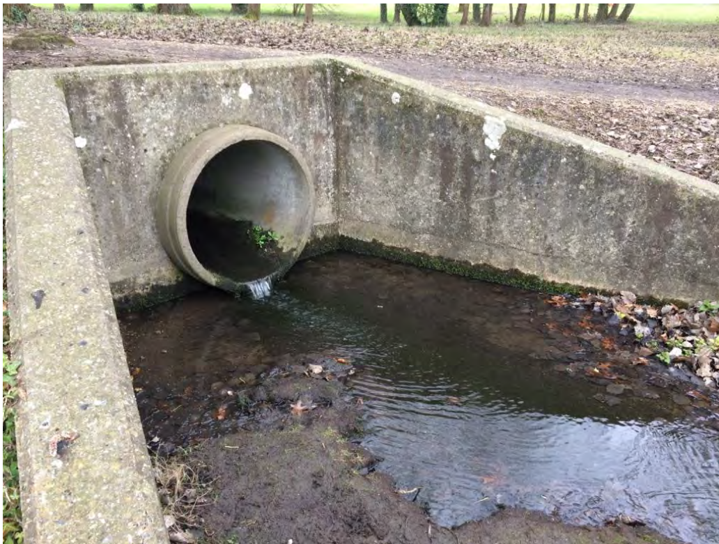
Photo 18 – Detail of Discharge Consented drainage (surrendered) identified 286m NE of site in Envirocheck report.
