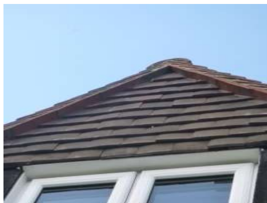
8. Slight gap under hanging tiles to the front of the house.
