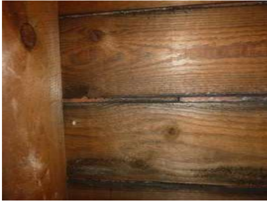
13. Gaps visible between the wooden sarking.
