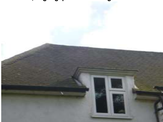
5. Uneven roof tiles just below the hip tiles to the rear of the house.
