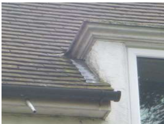
7. Lead flashing tight around the rear dormer window and large open gap at junction with the roof.
