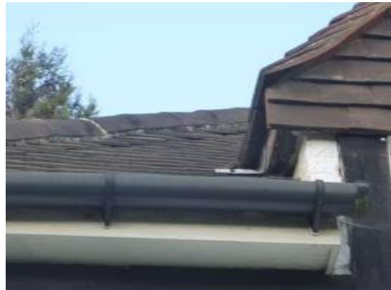
4. Uneven roof tiles just below the hip tiles to the front of the house.
