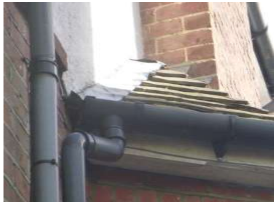
6. Lead flashing lifted around the sides of the chimney.
