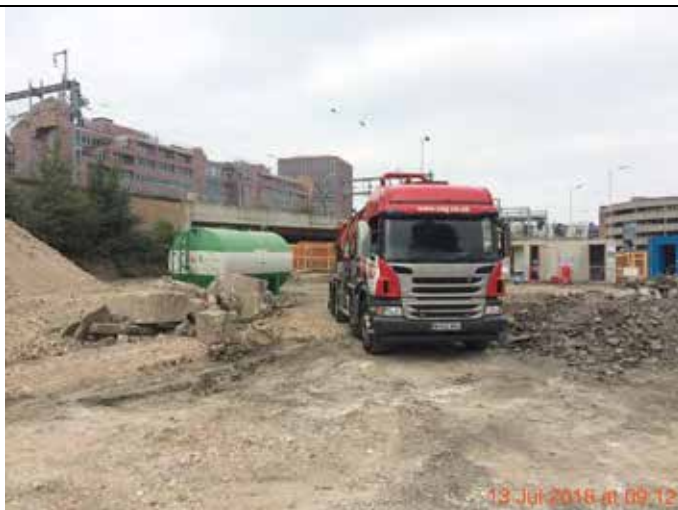
Photograph 51 – Vacuum tanker attendance to remove contaminated water / oil from the on-site header tank.
