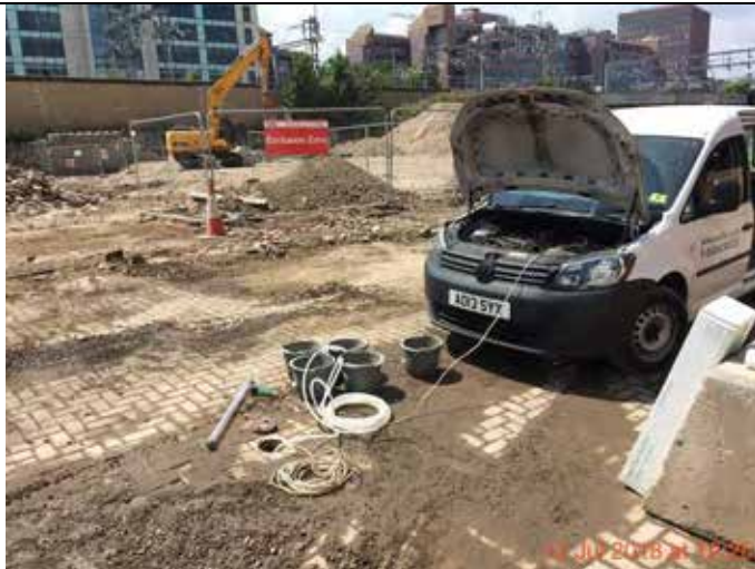
Photograph 49 – WaSP submersible pump used to purge the required volume from each well / sump.
