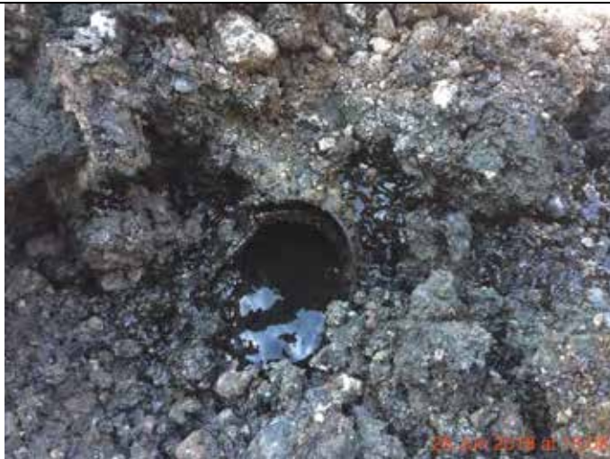
Photograph 20 – The deep surface water drainage pipe located within STP11 was chased back and free phase product was present throughout the entire length.
