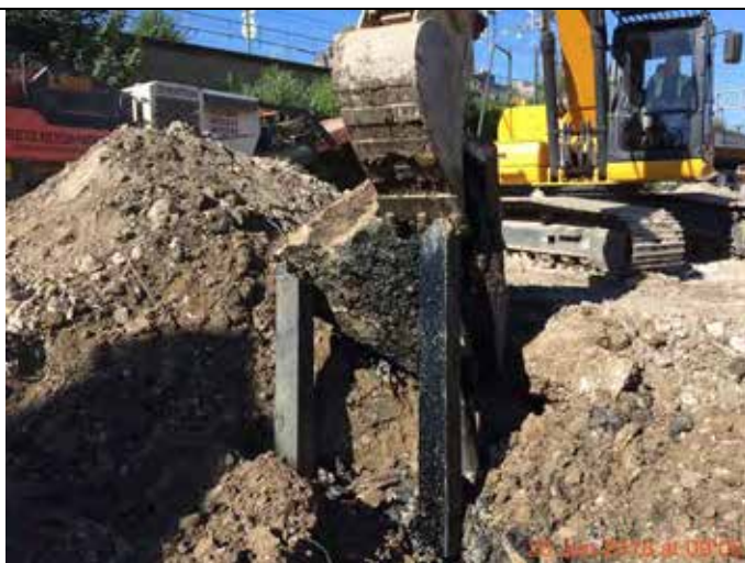
Photograph 15 – Piles removed from ground with accumulations of free phase product found there.
