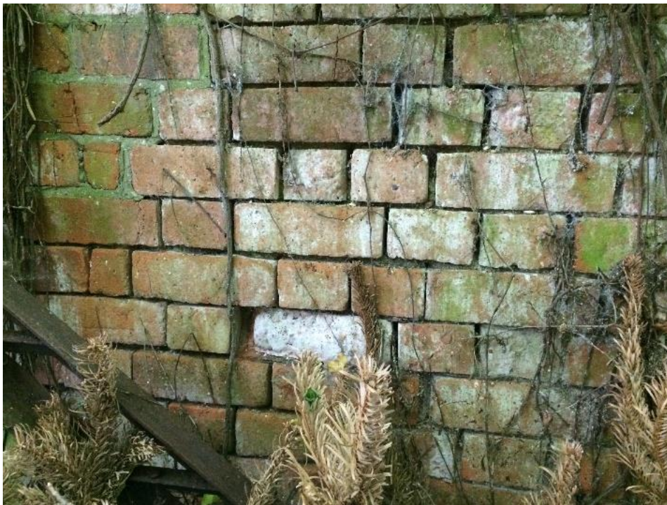
Photo 2: TN1 gaps in bricks
