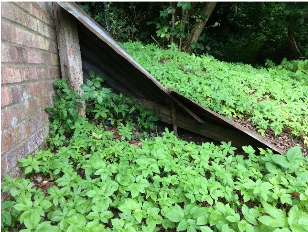
Photo 11: TN9 collapsed corrugated iron revetment with ground elder
