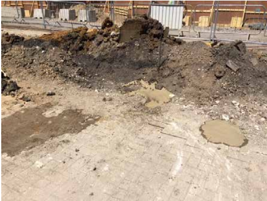
Photo 19. Grout appearing at surface on failed attempts (03/07/2018)
