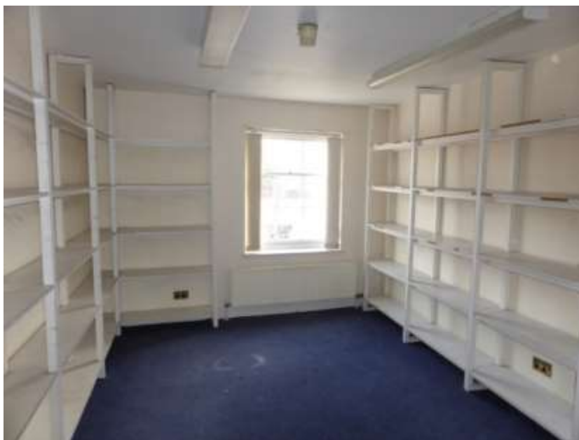
Figure 37: Blocked sash window opening to the left in S1
