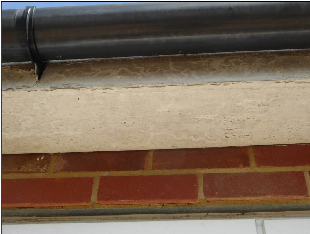
Figure 6. Soffits and fascias, 6 Courtenay Drive, Caversham. 26.07.18
