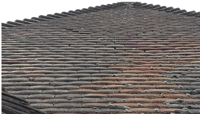
lifts in the front elevation roof space
