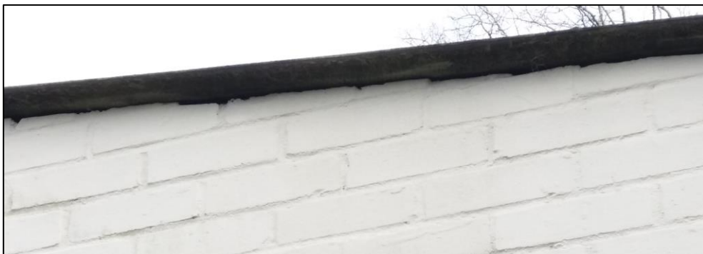
Figure 10 – gable end showing gap between wall and corrugated asbestos fibre board
