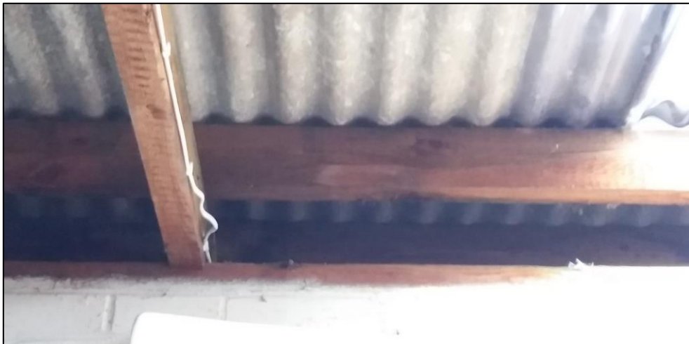
Figure 5 – showing gap at top of wall dividing the garage
