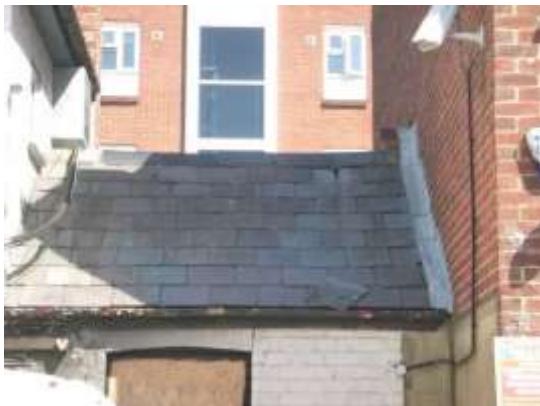
5. The low level roof in the south eastern corner showing slipped slate.
