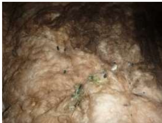
14. Scattered rat droppings on the fibre glass throughout the void.
