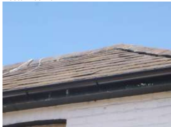
6. Slightly lifted slates on the hipped roof at the south eastern corner.
