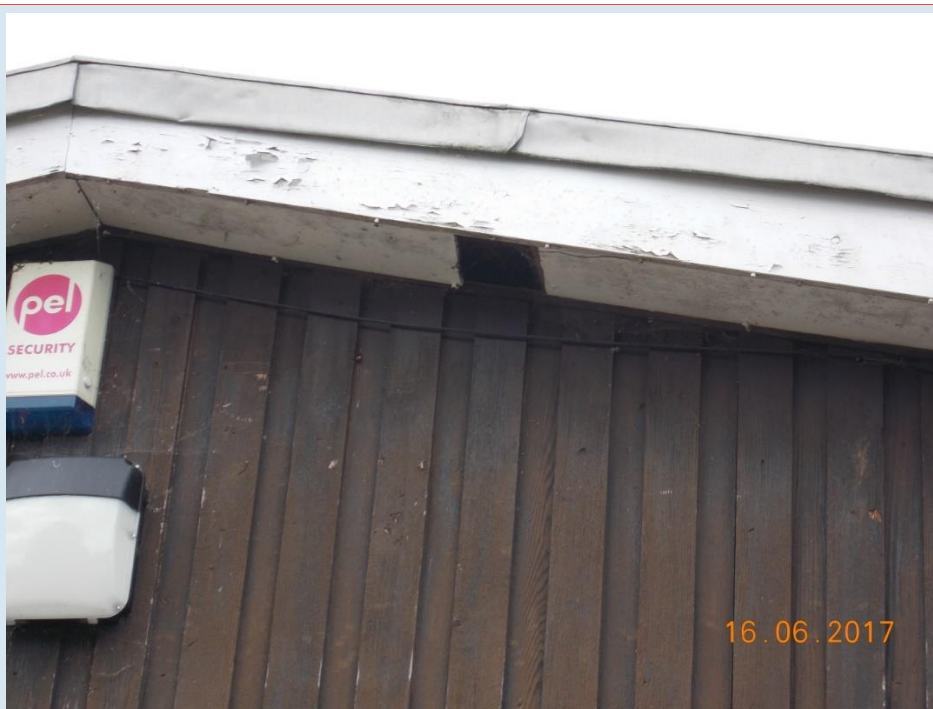
Gap in barge board (T2)
