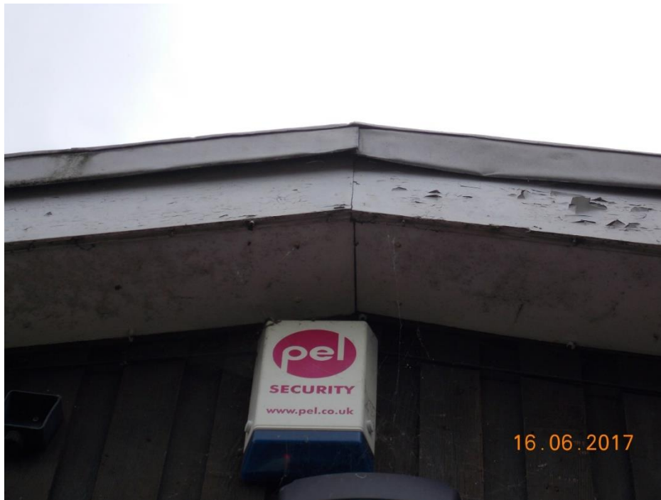
Gap between barge board and roof flashing (T3)
