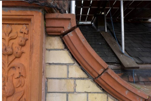
Photo 20b: Details of Copings to the front parapet wall The photo shows the lifting of the copings to No 15(neighboring building) with the creation of open joints that will be prone to water penetration and associated problems of damp and decay.
