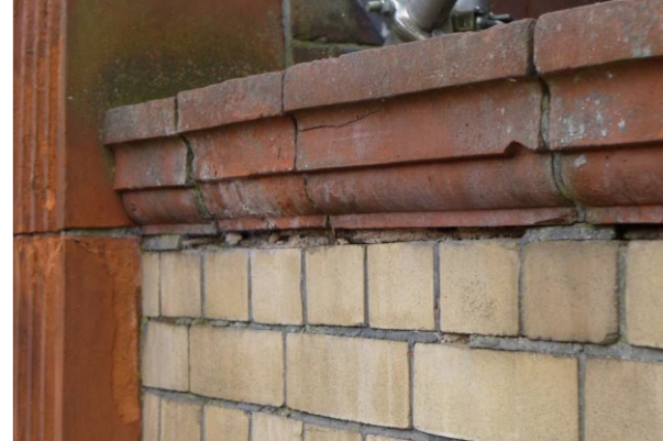
Photo 20a: Details of copings to the front parapet wall Photo shows the copings to No.17; note cracking to a coping, water staining and deterioration to the mortar of the bedding joint. There is a high risk of imminent failure
