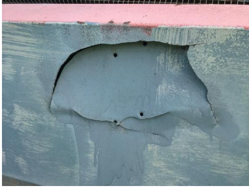
Plate 1: Building 1 - Damaged Metal Gutter
