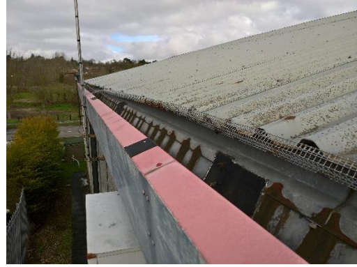
Plate 2: Building 1 – Thin Metal Gutter
