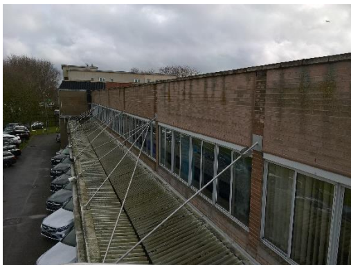
Plate 3: Building 2 – Weep Holes above Windows
