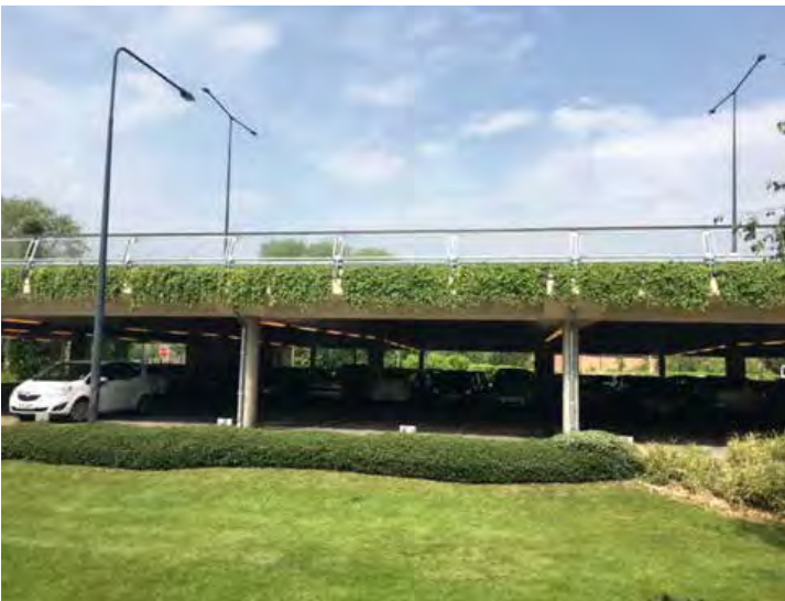
Figure 7. Example of ivy growing over and hanging down from a structure
