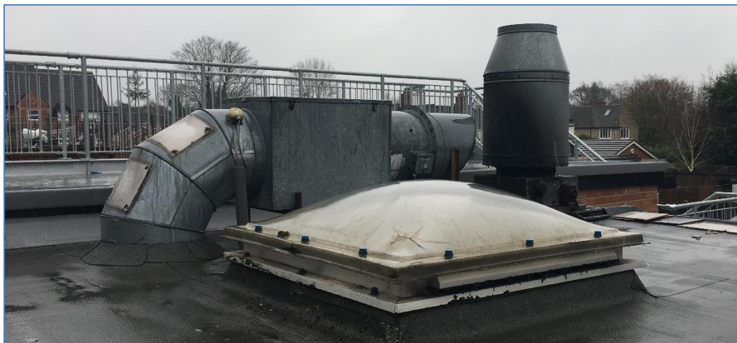
Extract equipment on neighbouring rear flat roof
